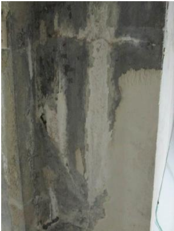
Image 1: Crack in the Pool Structure
