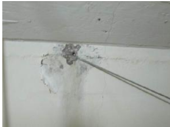
Image 65: Old Deck Plate Wiring at Shallow End
