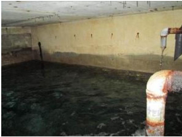
Image 90: Interior of Surge Tank
