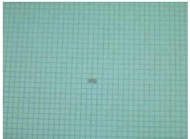
Image 12: Missing Tiles in the Shallow End
