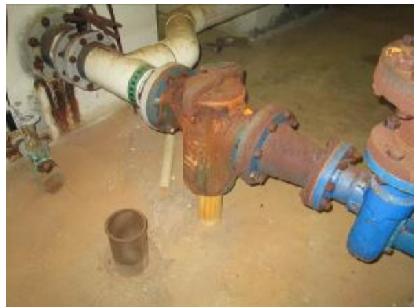
Image 79: Corroded Hair and Lint Strainer and Reducer
