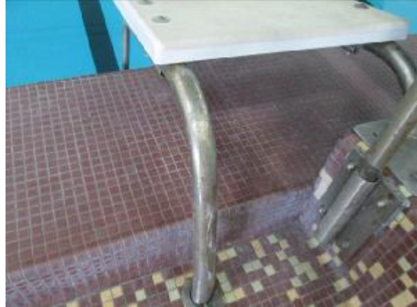
Image 49: Mild Corrosion on Stainless Steel Starting Block Posts
