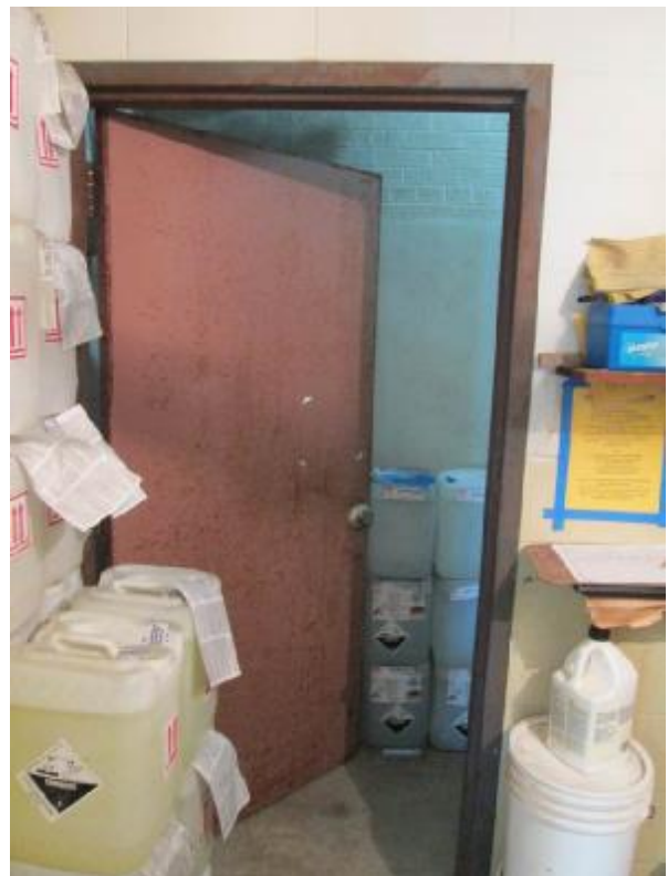
Image 101: Chemical Storage and Corroded Door and Frame
