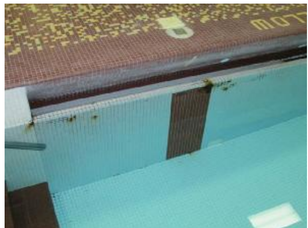
Image 14: Corrosion at the Water Line Handhold
