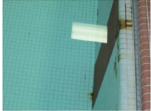
Image 16: Corrosion at the Water Line Handhold
