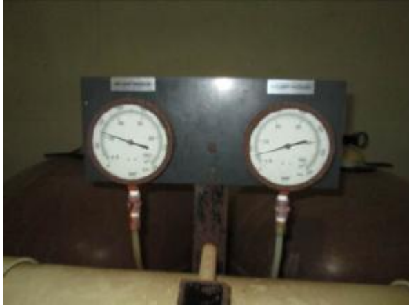
Image 86: Influent and Effluent Pressure Gauges
