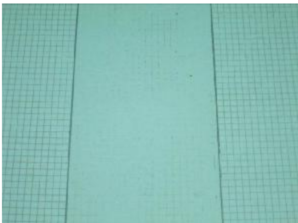
Image 13: Lime Build-Up and Missing Grout
