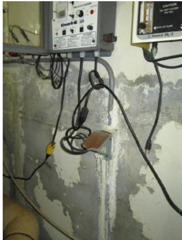
Image 110: Water Chemistry Controller Wiring Connections
