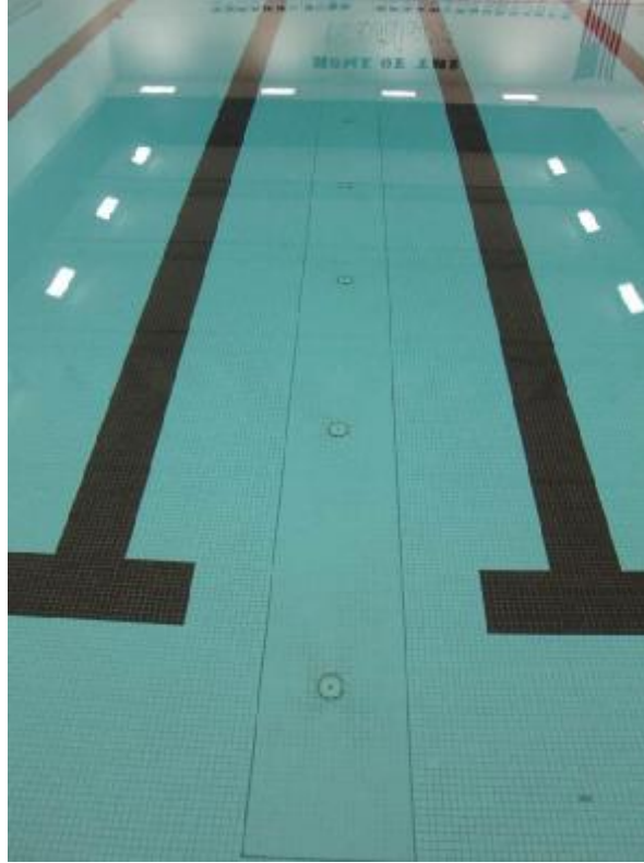
Image 26: Pool Floor Return Inlets
