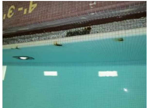
Image 22: Metallic Gutter Dropout and Handhold Corrosion
