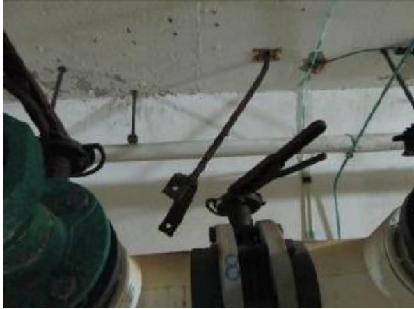
Image 74: Example of Corroded Pipe Hanger Failure
