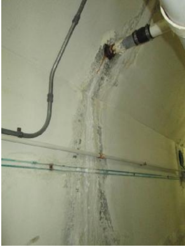
Image 3: Pool Leak Emanating from Pool Piping
