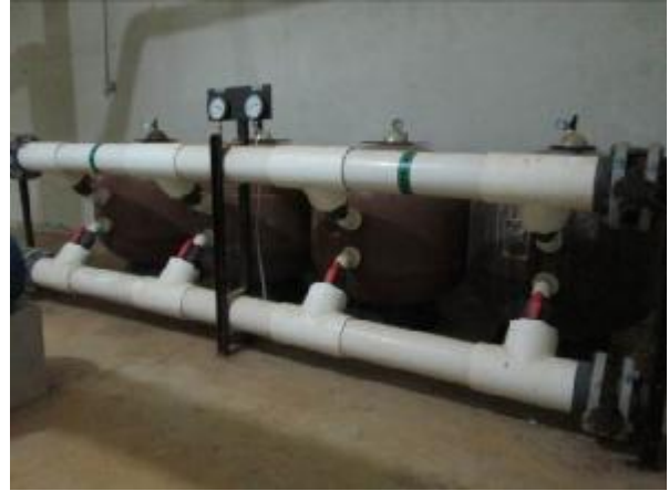
Image 87: Schedule 40 PVC Filter Face Piping
