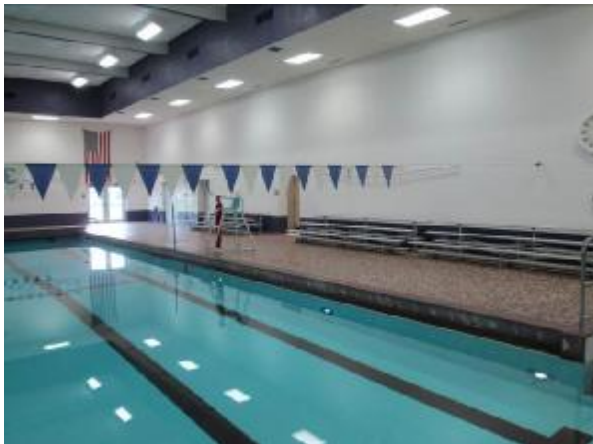
Image 21: Rollout Perimeter Overflow Gutter along the Length of the Pool
