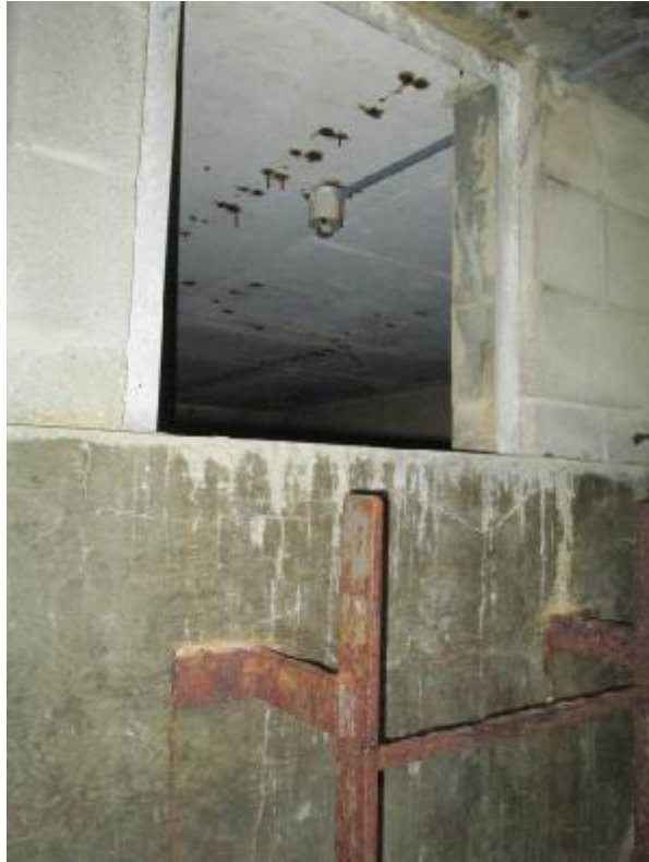
Image 94: Surge Tank Access and Ladder
