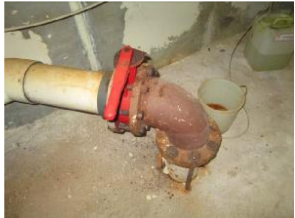
Image 71: Main Drain Suction Piping
