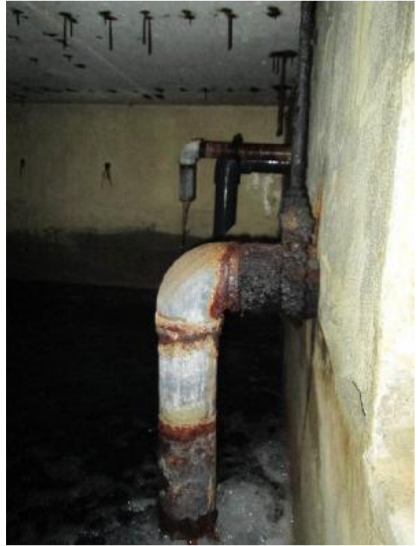
Image 112: Domestic Water Coming into Surge Tank
