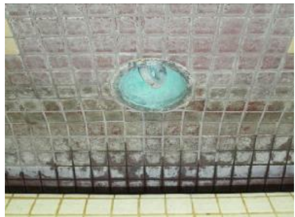
Image 31: Safety Rope Anchor
