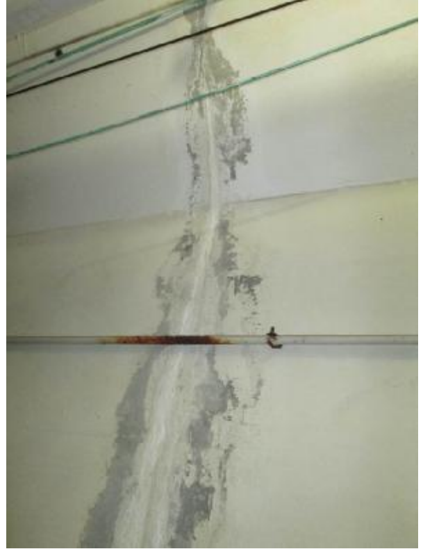
Image 4: Vertical Crack in the Pool Structure
