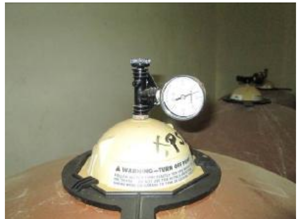
Image 85: Filter Tank Pressure Gauge
