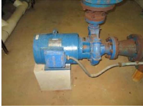
Image 80: Recirculation Pump and Base
