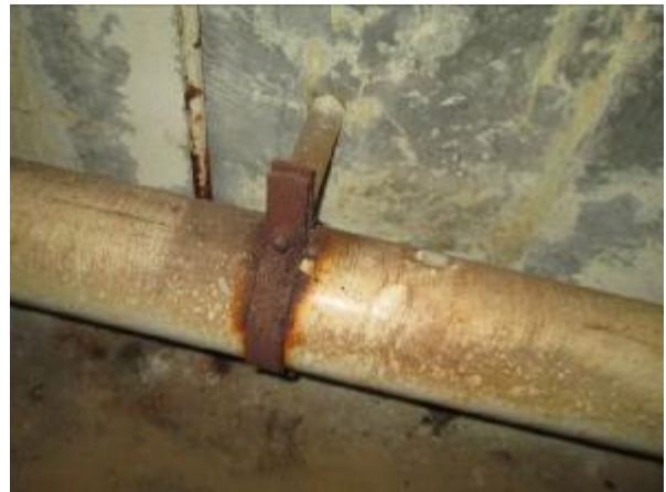
Image 73: Corroded Pipe Support
