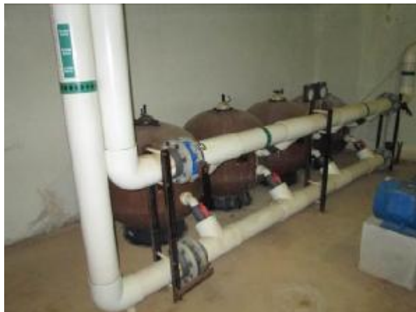
Image 84: High Rate Sand Filter Tanks
