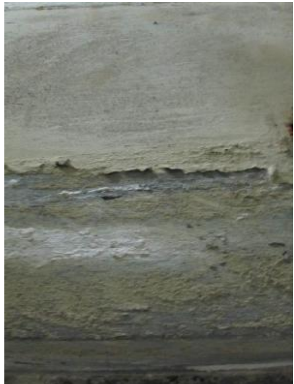
Image 2: Crack in the Pool Structure
