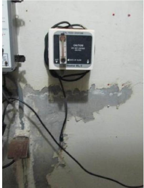
Image 99: Abandoned CO 2 Feed System
