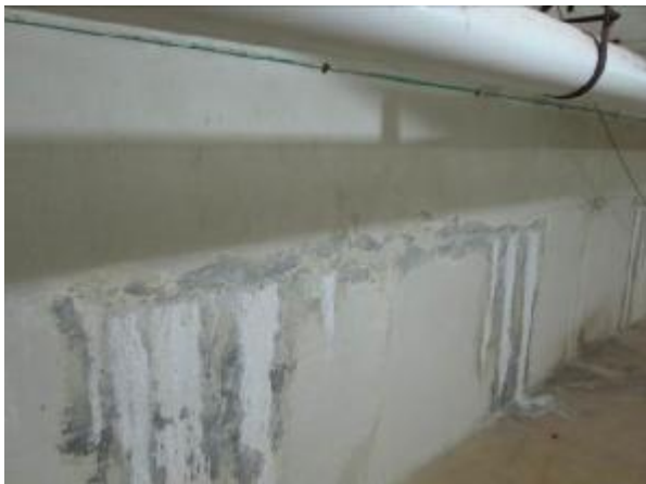
Image 9: Crack in the Pool Structure
