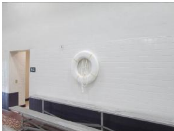
Image 55: Wall Mounted Ring Buoy with Extension Rope
