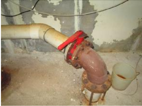
Image 88: Main Drain Suction Butterfly Valve
