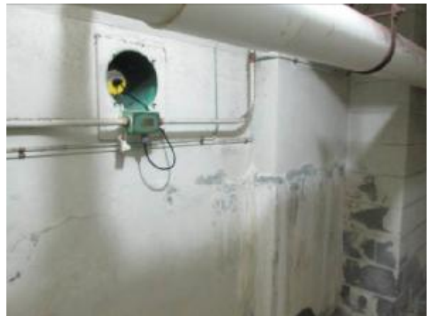
Image 10: Crack in the Pool Structure
