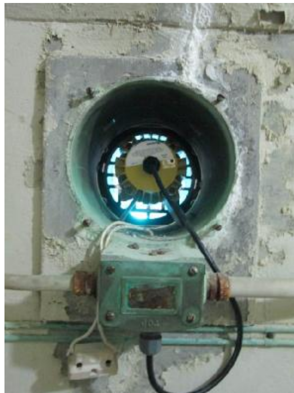
Image 29: Dry Niche and Backside of Underwater Light
