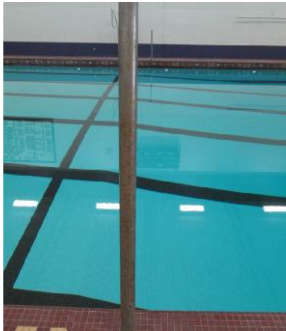
Image 53: Corrosion on Stanchion Post
