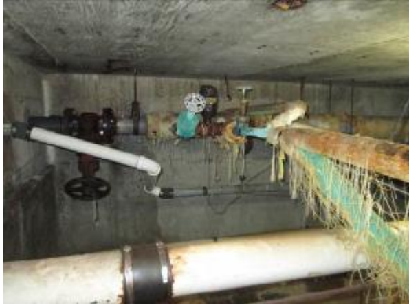
Image 111: Domestic Water to Pool System
