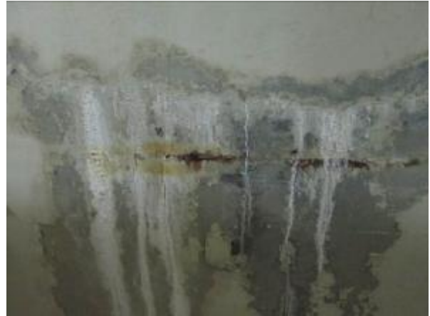
Image 6: Crack in the Pool Structure and Calcification
