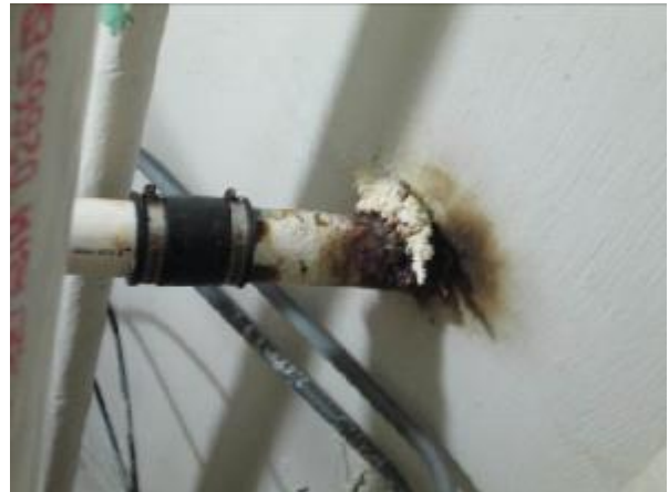
Image 77: Gutter Dropout Penetration
