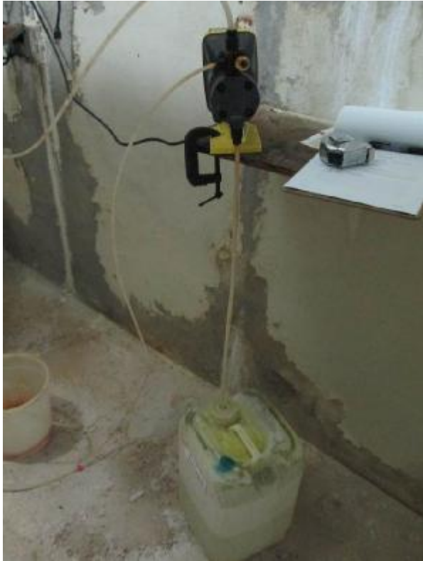
Image 98: Chemical Feed Pump and Tank
