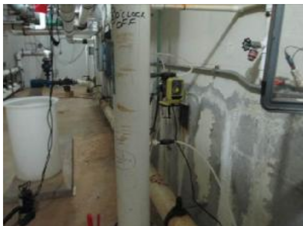
Image 96: Pool Chemical Feed Location
