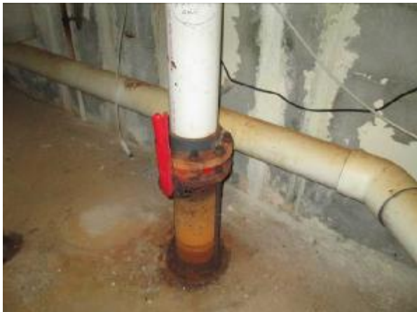
Image 72: Return Piping and Valve
