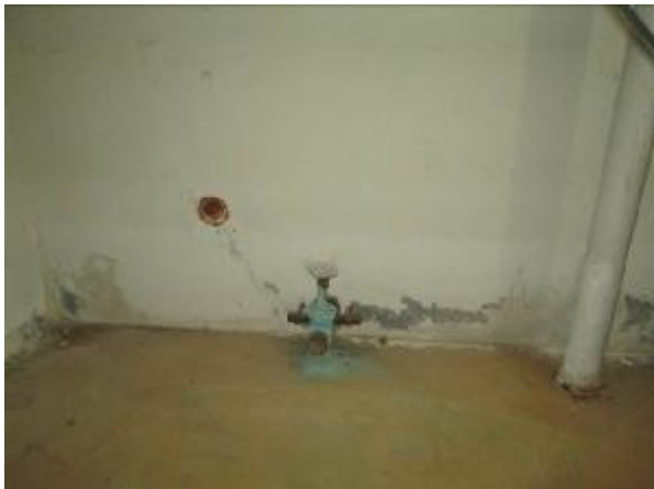
Image 92: Surge Tank Drain
