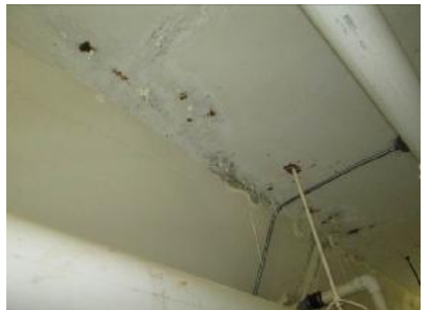
Image 20: Stalactites from the Underside of the Pool Deck
