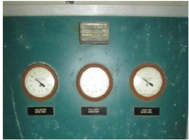
Image 91: Surge Tank Water Level Control and Heater Temperature Readouts
