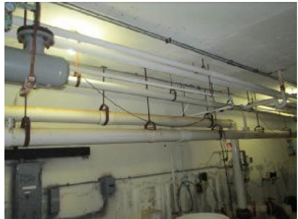
Image 67: Corroded Mechanical Room Pipe Hangers and Supports
