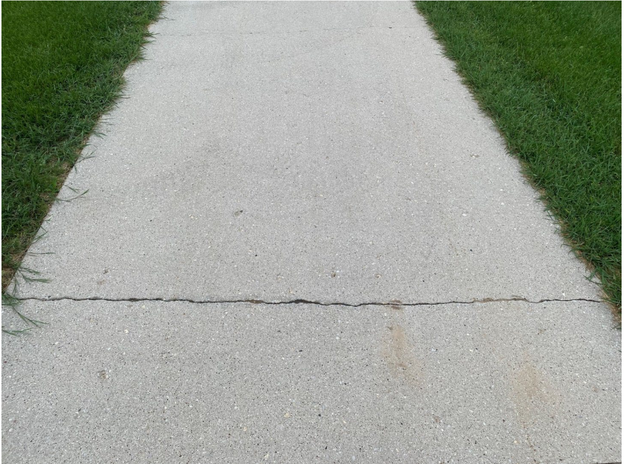
Figure 15: Horizontal crack in front center west sidewalk.
