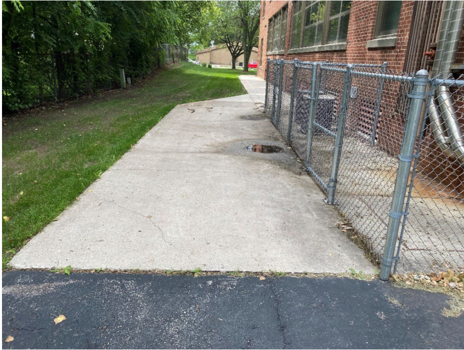
Figure 60: Cracking and settling in concrete slab on east side of school causing water to pool.
