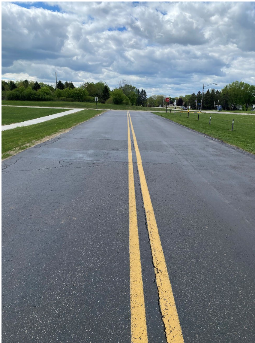
Figure 11: South portion of Access Drive in fair condition.
