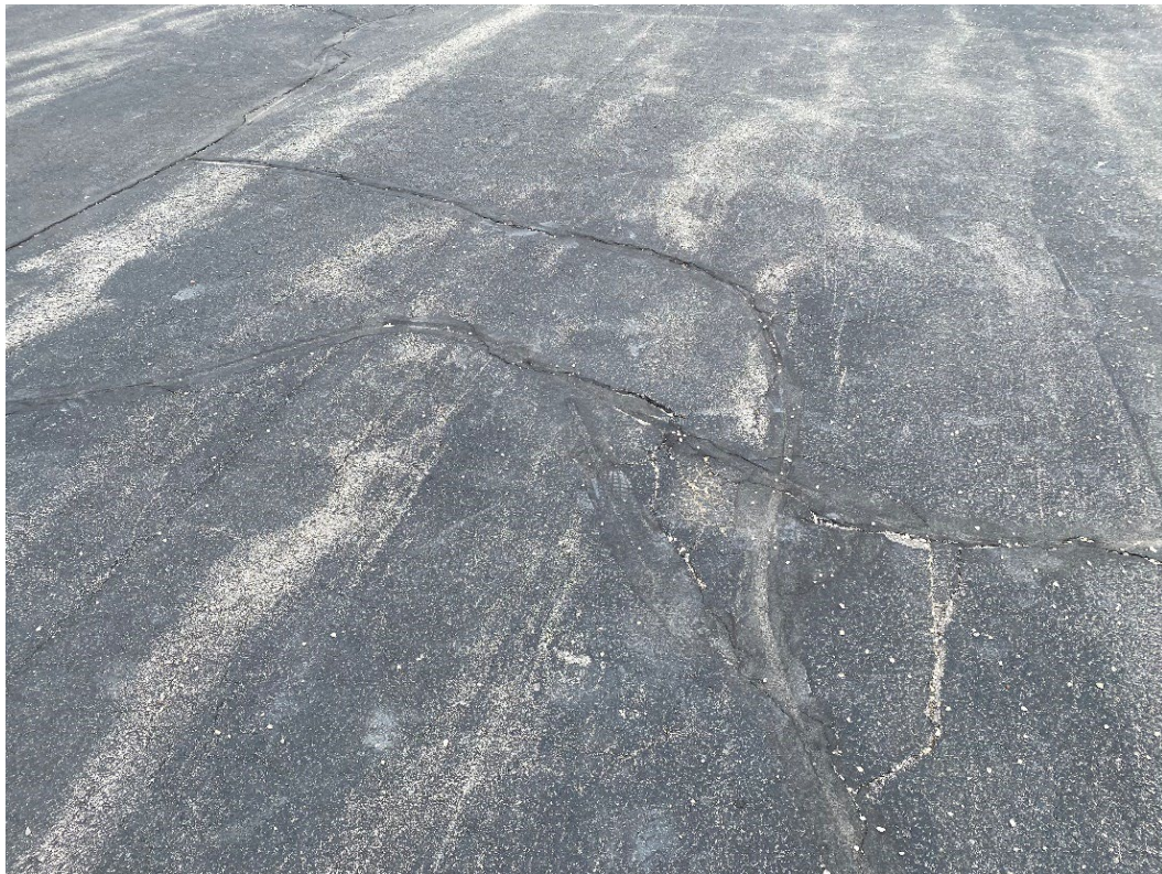
Figure 24: Cracks in play area surface
