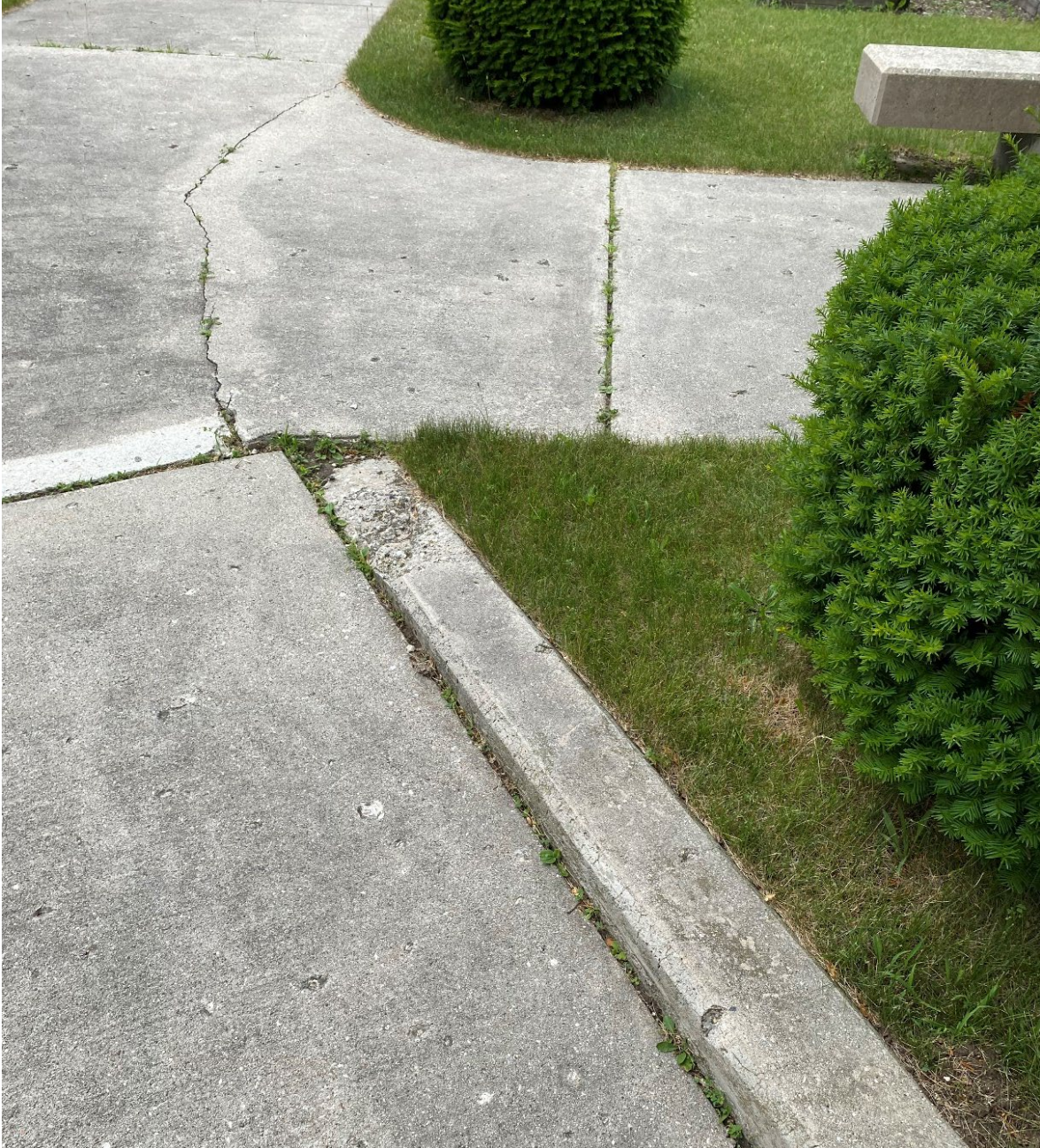
Figure 41: Cracking in sidewalk and deteriorating concrete retaining wall in courtyard.
