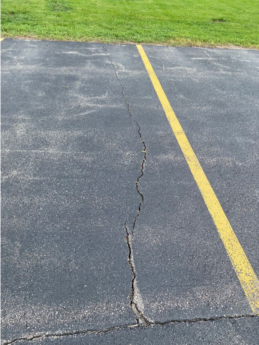
Figure 86: Longitudinal and transverse cracking in parking stalls in northwest parking lot.
