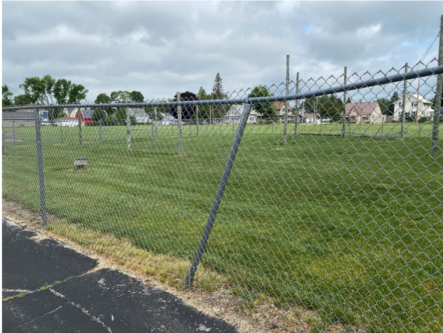
Figure 54: Fence surrounding climbing area falling over.
