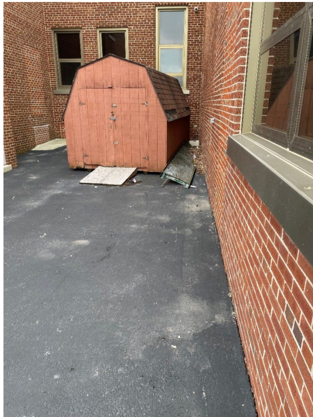
Figure 44: Deteriorating shed in back play yard.
