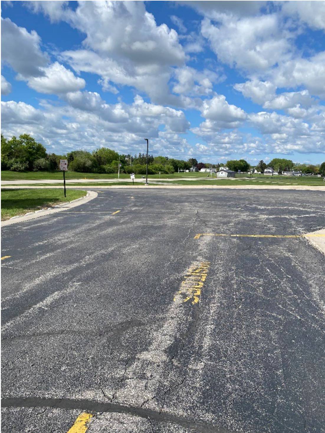
Figure 3: Faded pavement markings in Bus/Visitor Parking Loop.
