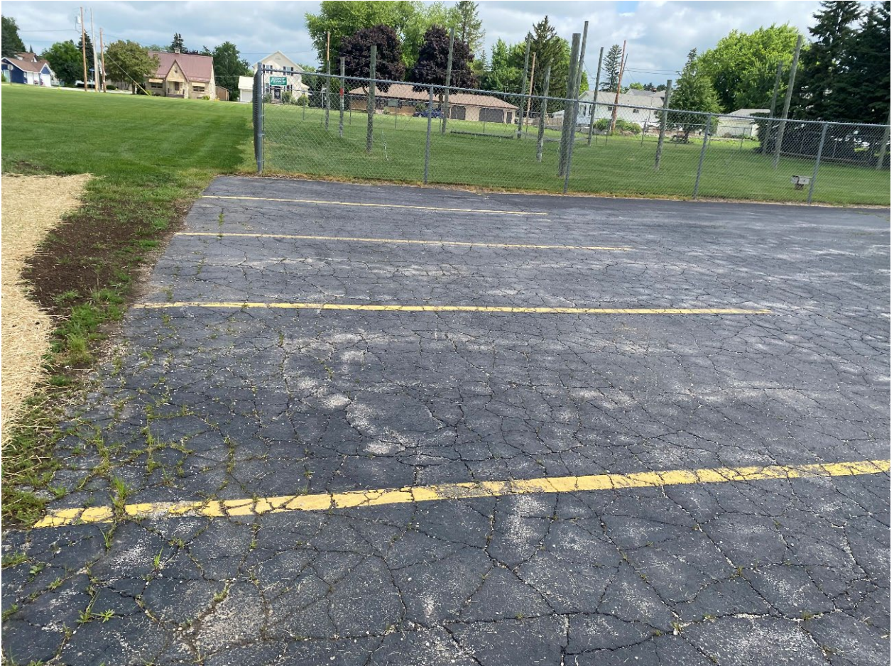
Figure 52: Northeast parking lot covered in alligator cracking.
