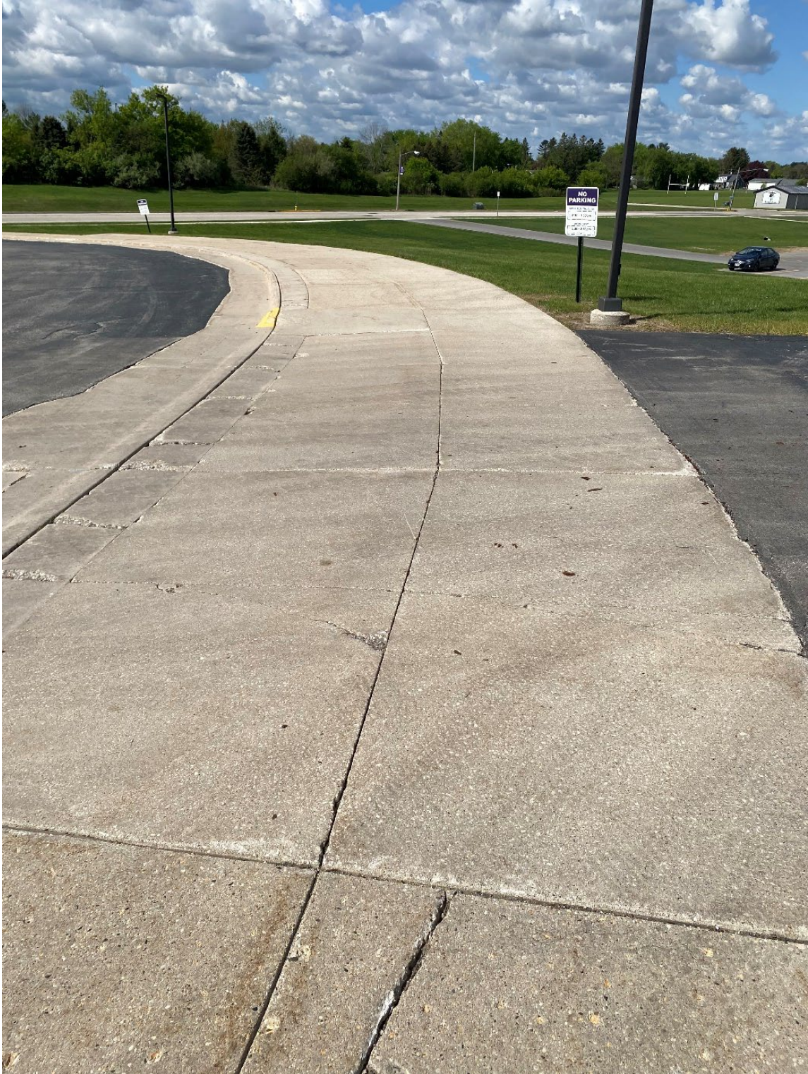
Figure 6: Cracked concrete sidewalk driveway apron into garbage dumpster area along Bus/Visitor Parking Loop.
