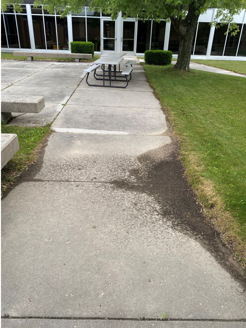
Figure 43: Accumulation of soil due to settling pavement in courtyard.
