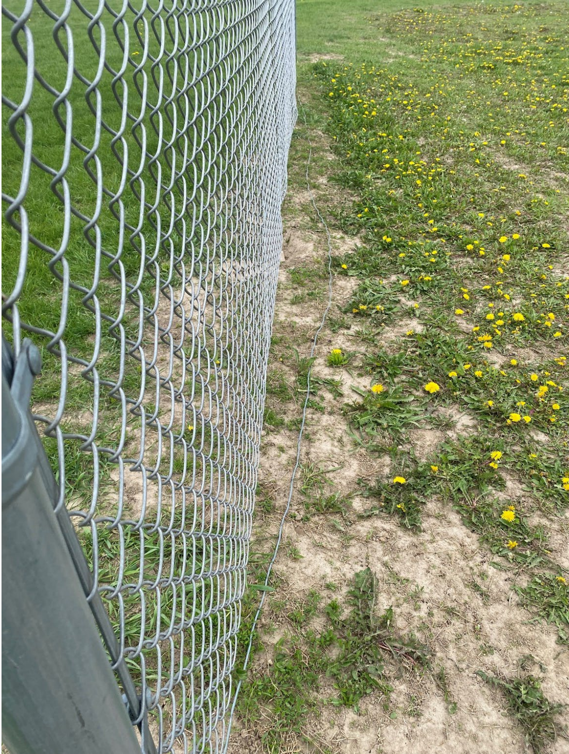
Figure 15: Broken fence with loose wire next to ball field
