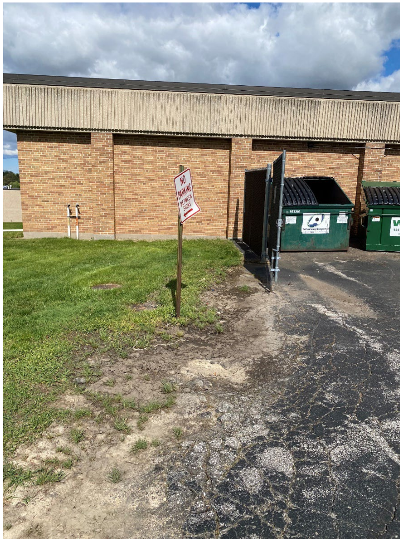
Figure 7: Significant edge cracking in Garbage Dumpster Parking Lot.
