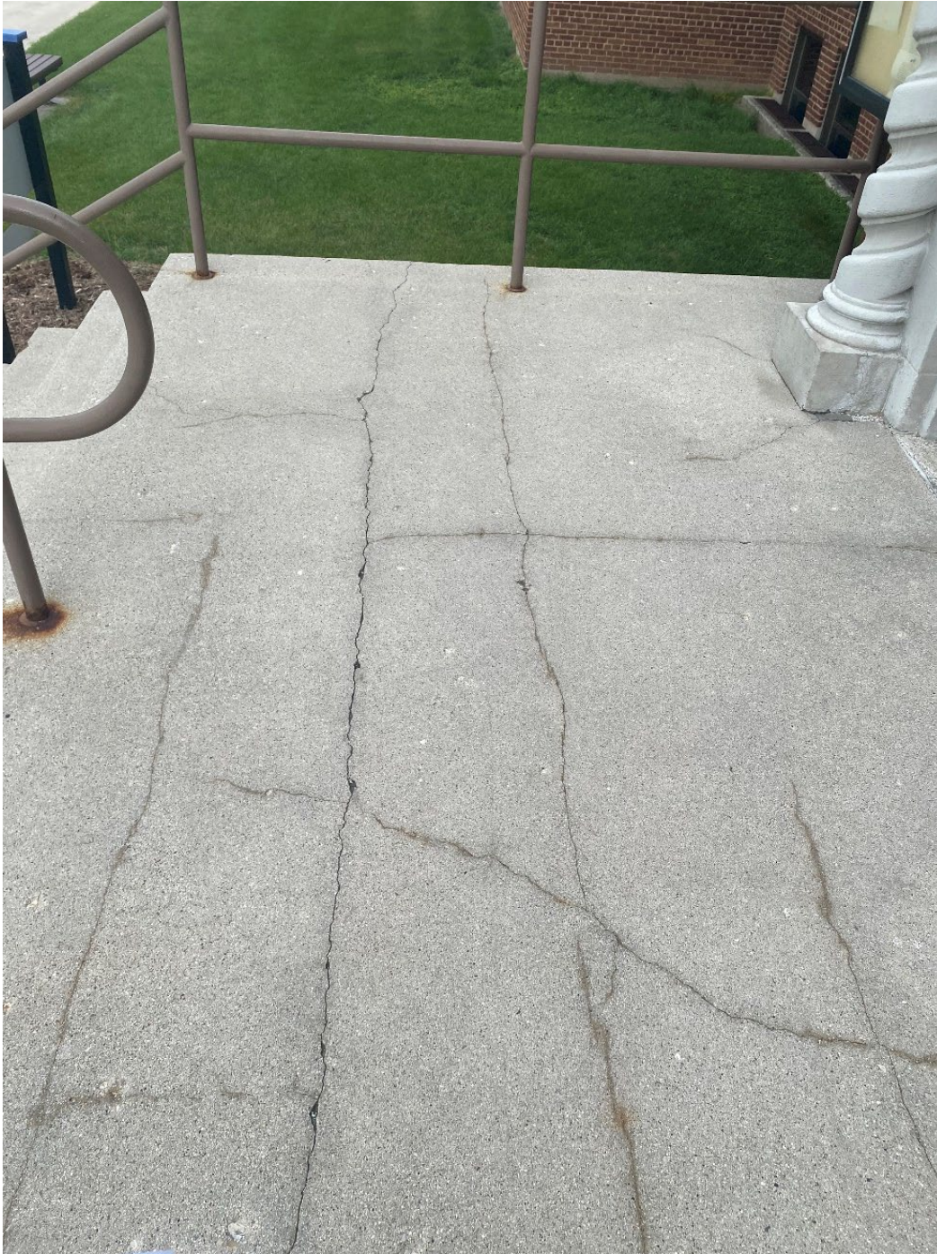
Figure 14: Top of front center west stair in poor condition.
