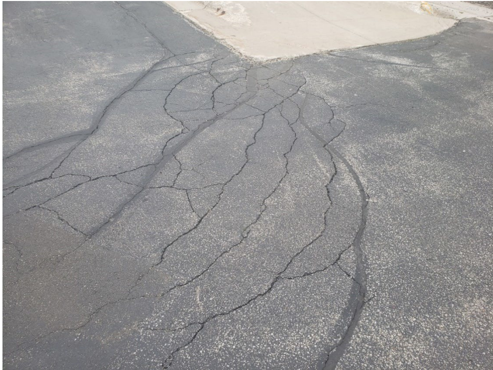
Figure 3: Cracked pavement on the North portion of West parking lot.
