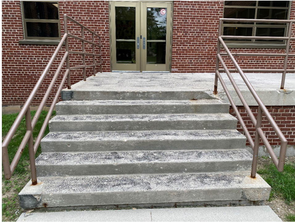
Figure 4: Front east stairs in poor condition.
