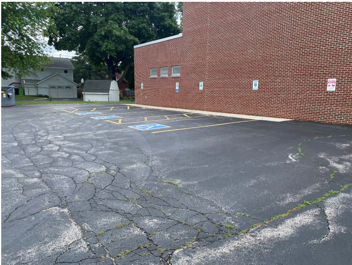
Figure 48: ADA parking area in poor condition due to alligator cracking.
