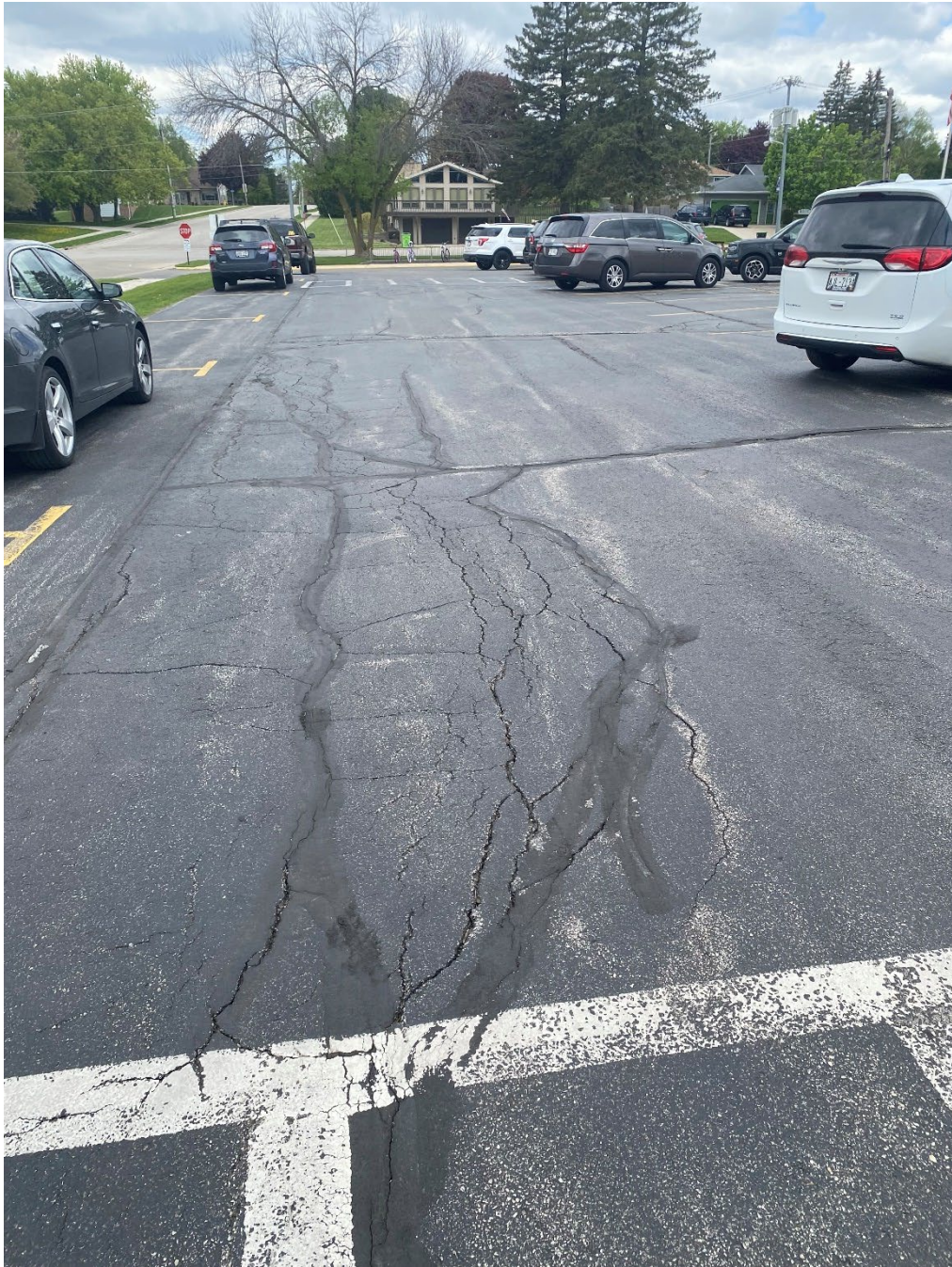
Figure 9: South parking lot cracking
