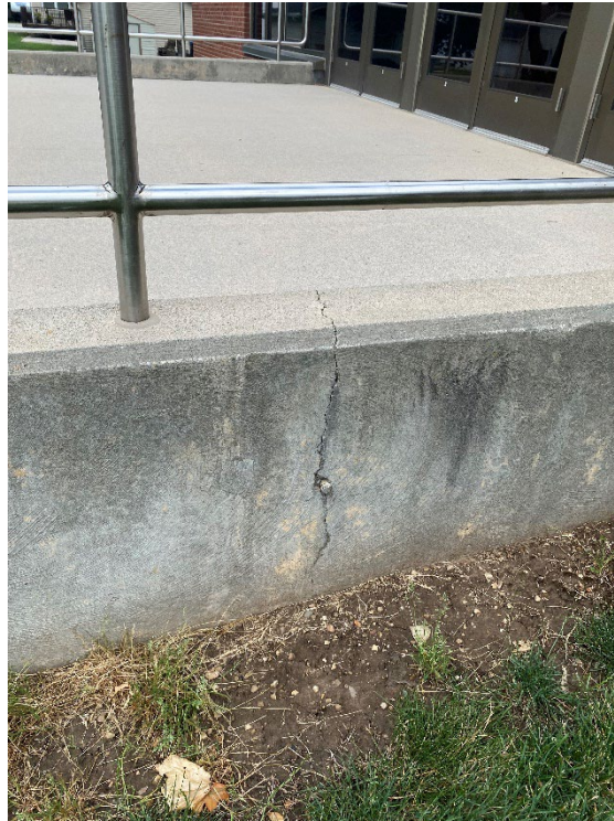
Figure 23: Crack in foundation of front west stairway.
