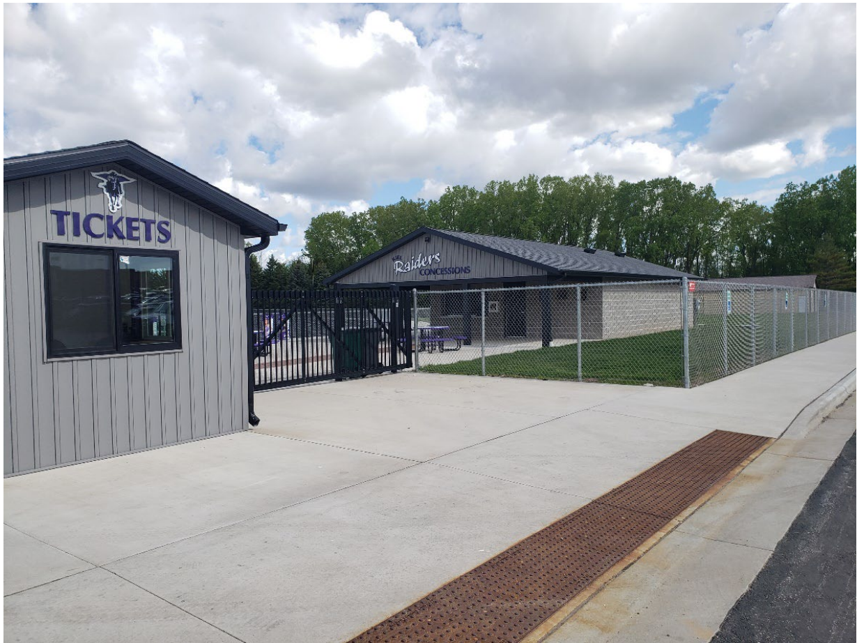
Figure 22: Rusted truncated dome in entrance to running track.
