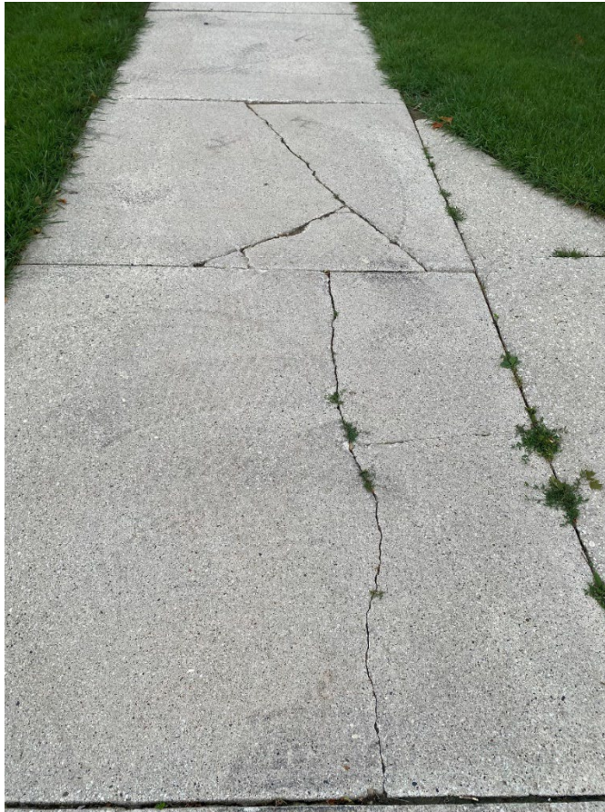
Figure 26: Severe cracking in front west sidewalk.
