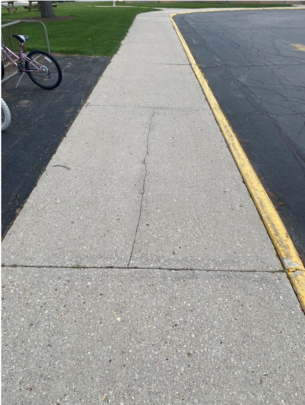
Figure 10: Crack in west sidewalk
