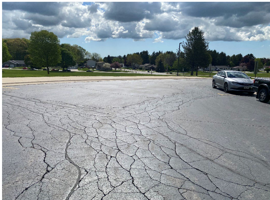
Figure 2: Alligator and block cracking in asphalt pavement in Bus/Visitor Parking Loop.
