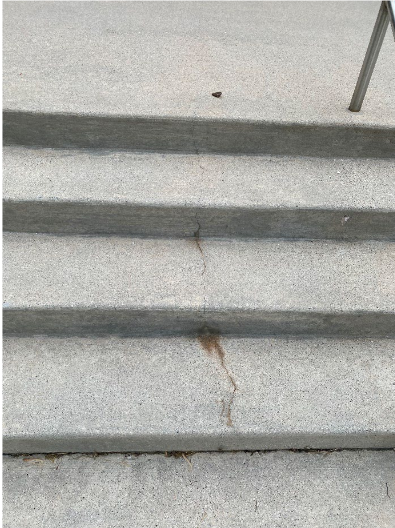
Figure 25: Crack on stairs of front west stairway.
