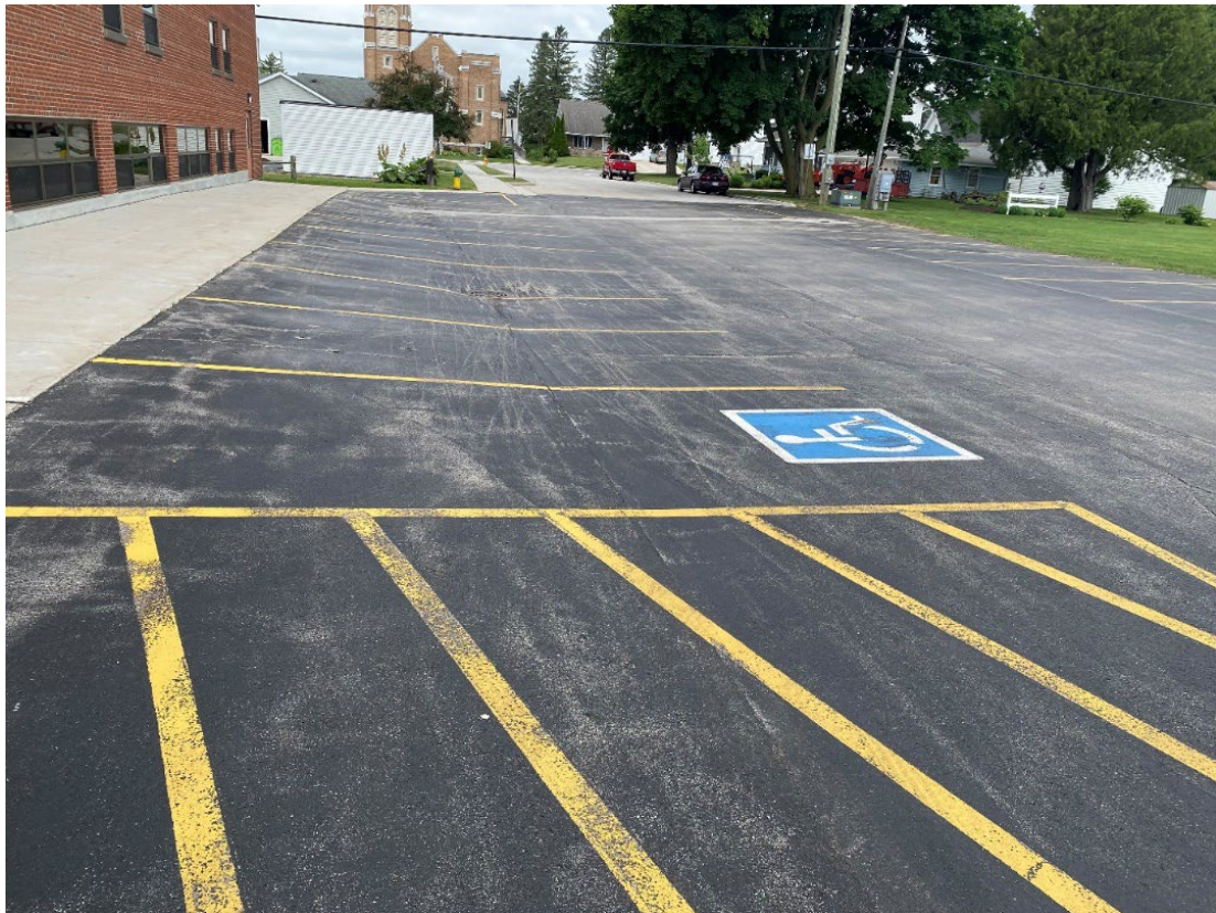
Figure 34: Longitudinal cracking in parking stalls in northwest parking lot.
