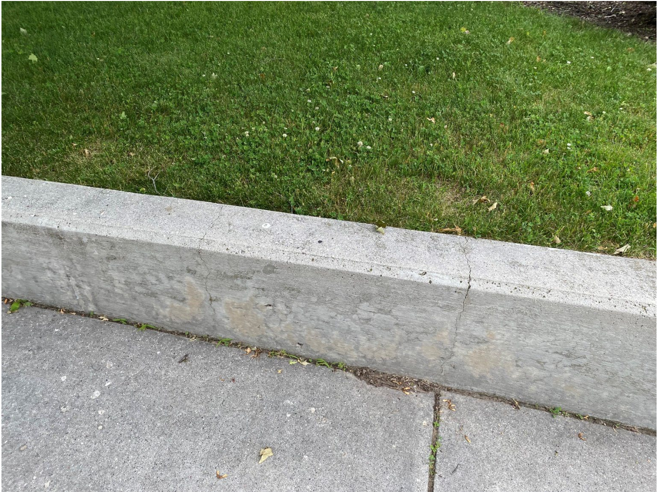
Figure 40: Cracking in concrete retaining wall in courtyard.
