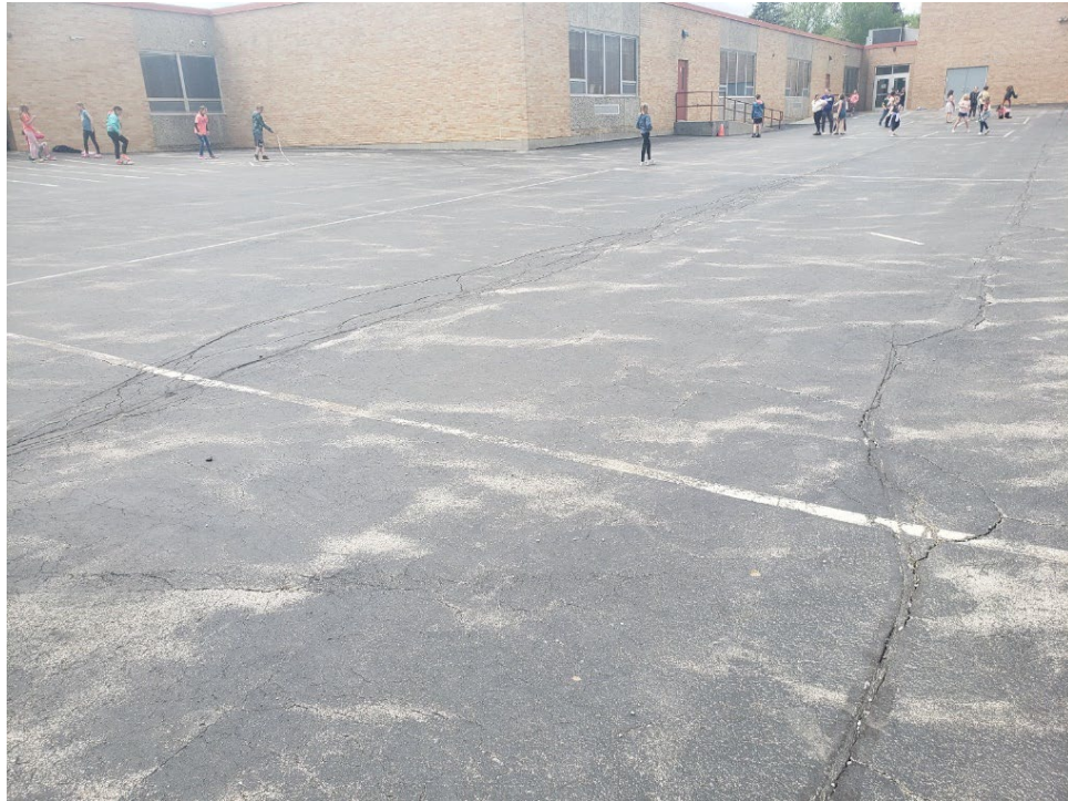
Figure 18: Longitudinal cracking and settling in the north play area
