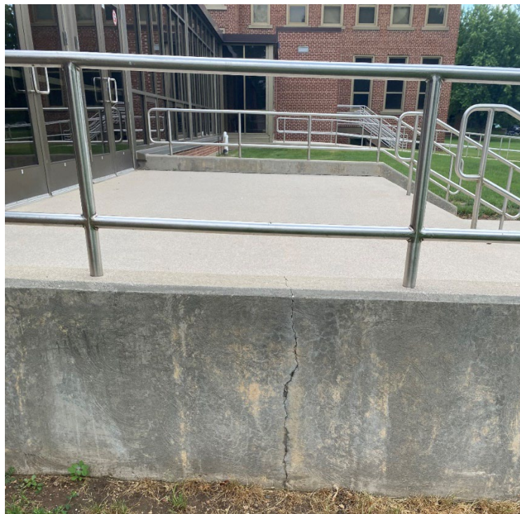
Figure 24: Another foundation crack on front west stairs.
