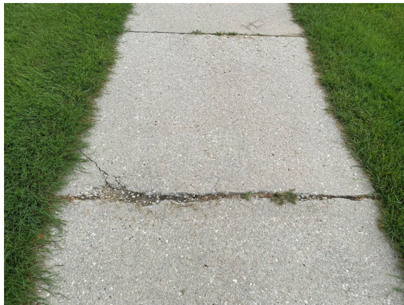
Figure 29: Deteriorating concrete on front west sidewalk.
