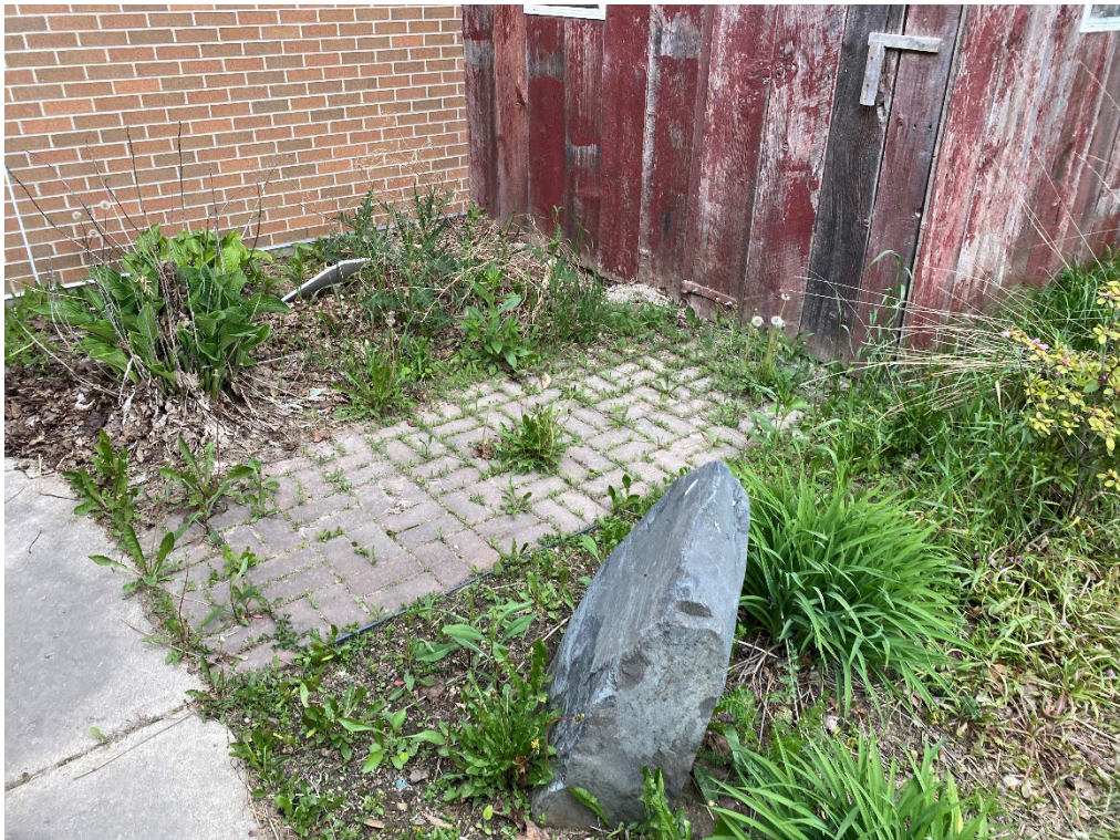
Figure 19: Overgrown pavers in front of small shed near goat pen on north side of school
