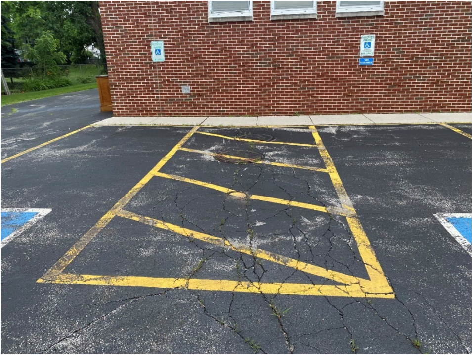
Figure 50: Alligator cracking and worn pavement markings in back east ADA stalls.
