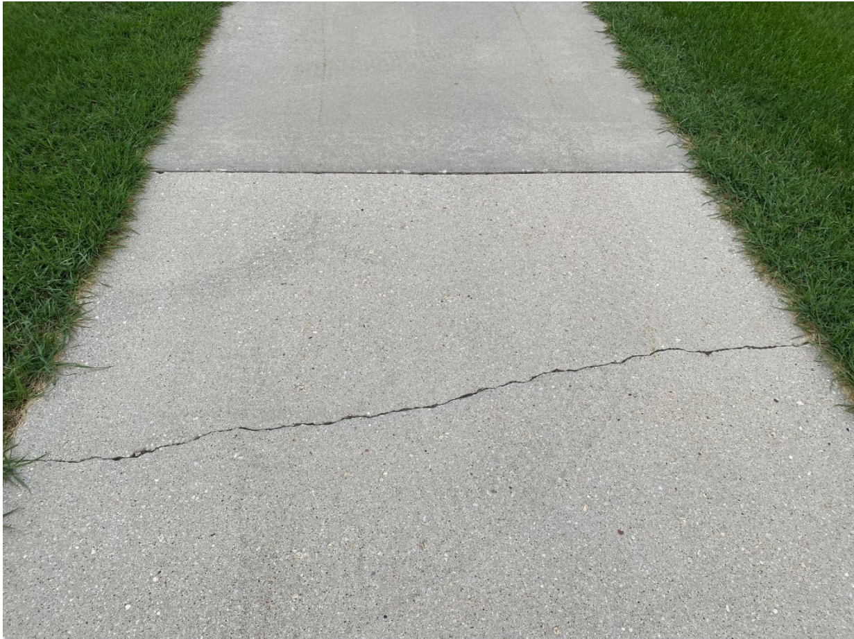
Figure 16: Diagonal crack in front center west sidewalk.
