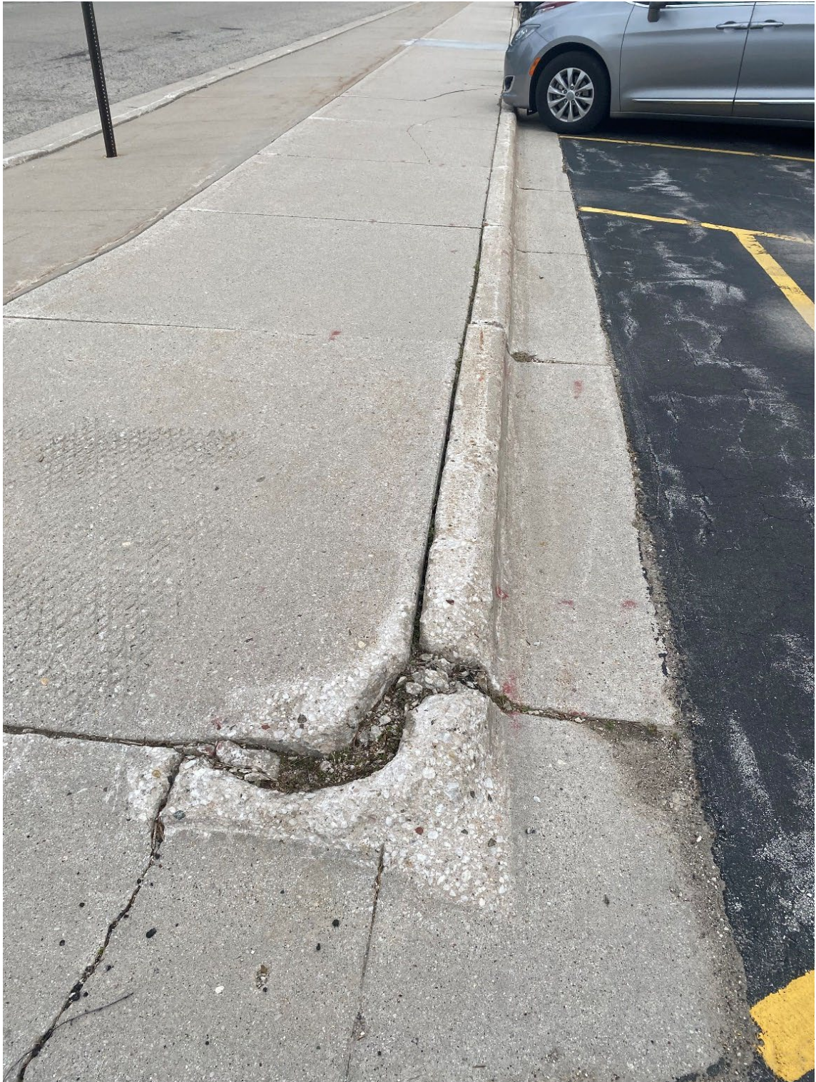
Figure 6: Deteriorated curb near south-west driveway apron
