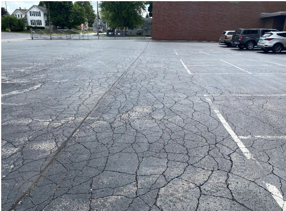
Figure 42: Alligator cracking throughout back play yard.
