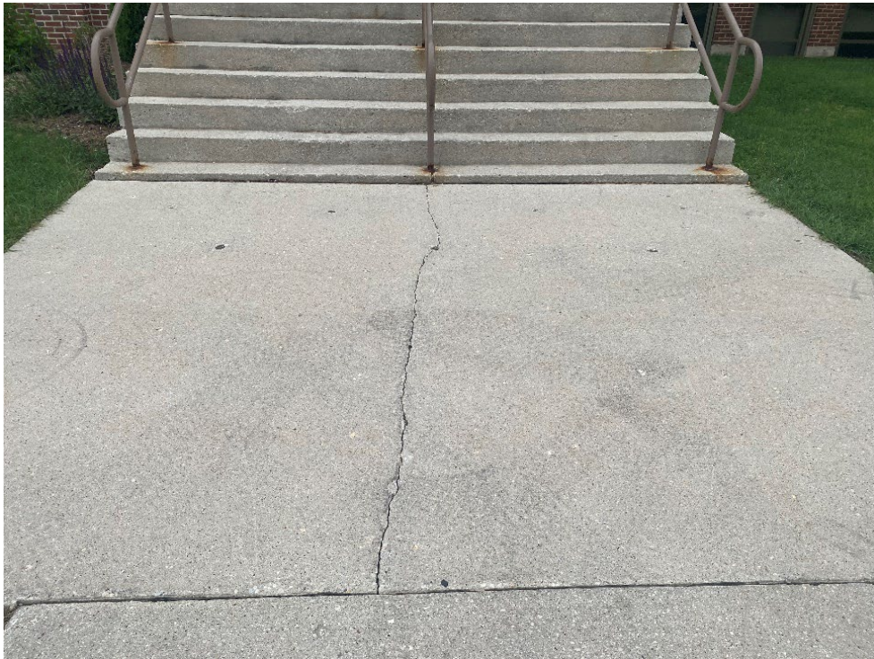
Figure 9: Vertical crack in concrete slab at bottom of front center east stairs.
