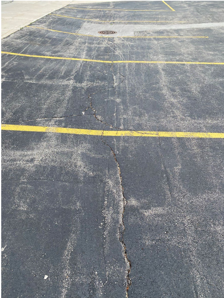
Figure 75: Longitudinal cracking in northwest parking lot.
