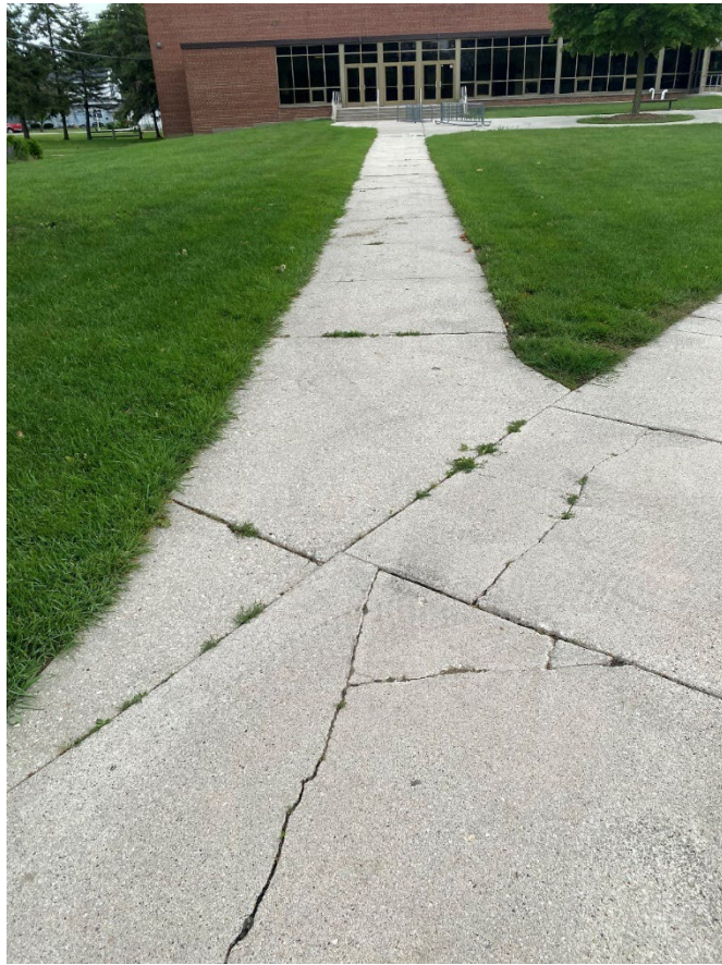
Figure 28: Cracking in front west sidewalk.
