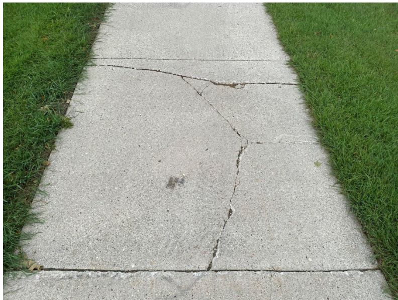
Figure 27: Additional cracking in front west sidewalk.
