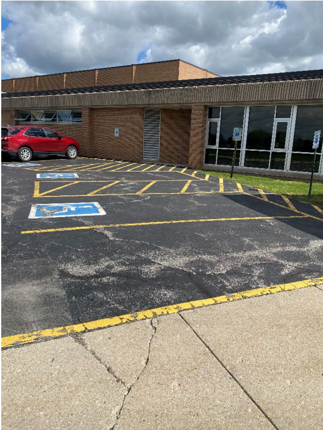
Figure 8: Pavement markings and signposts in poor condition in the Garbage Dumpster Parking Lot.
