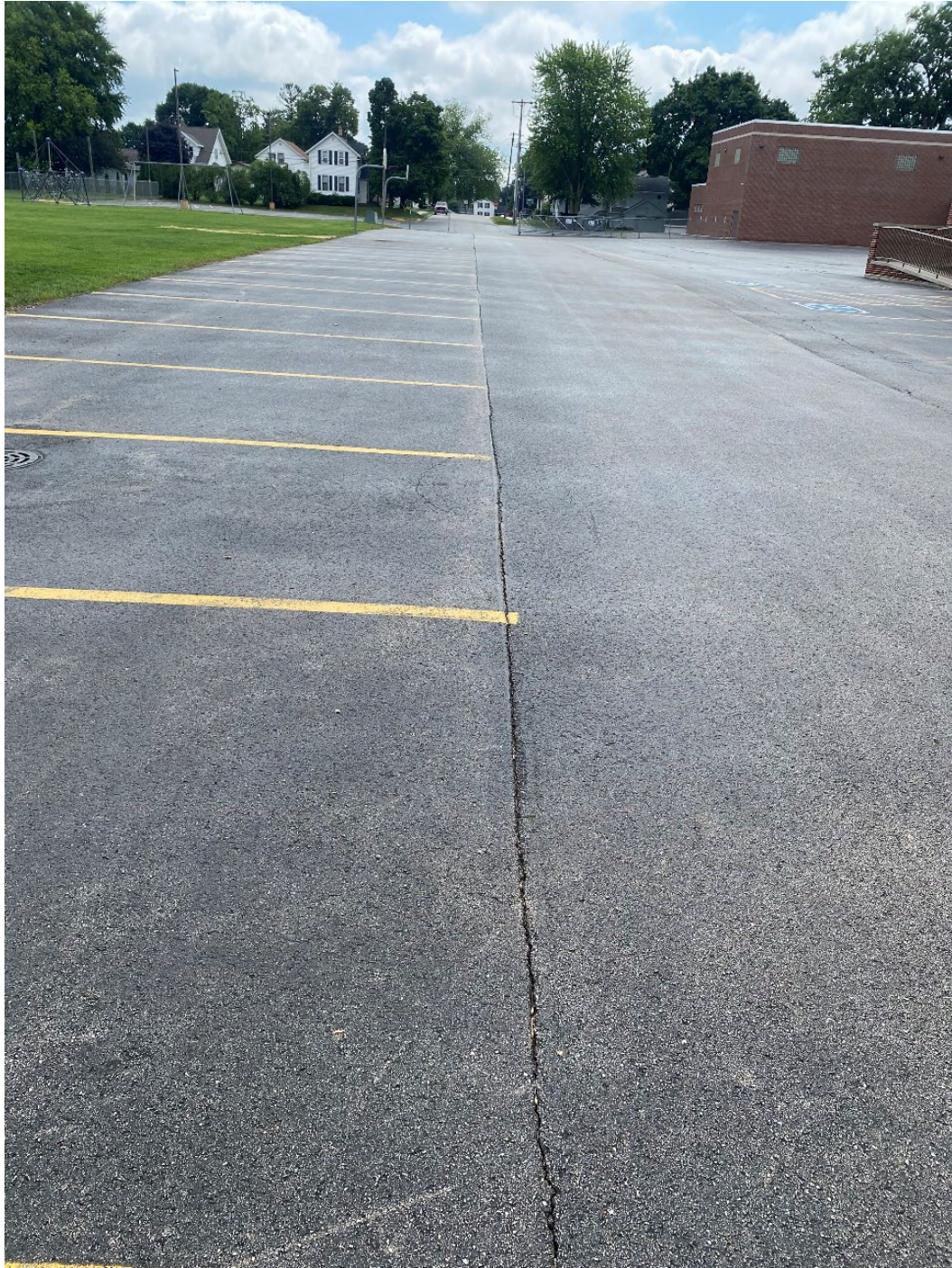
Figure 38: Newer pavement in drive lane of northwest parking lot in fair condition.
