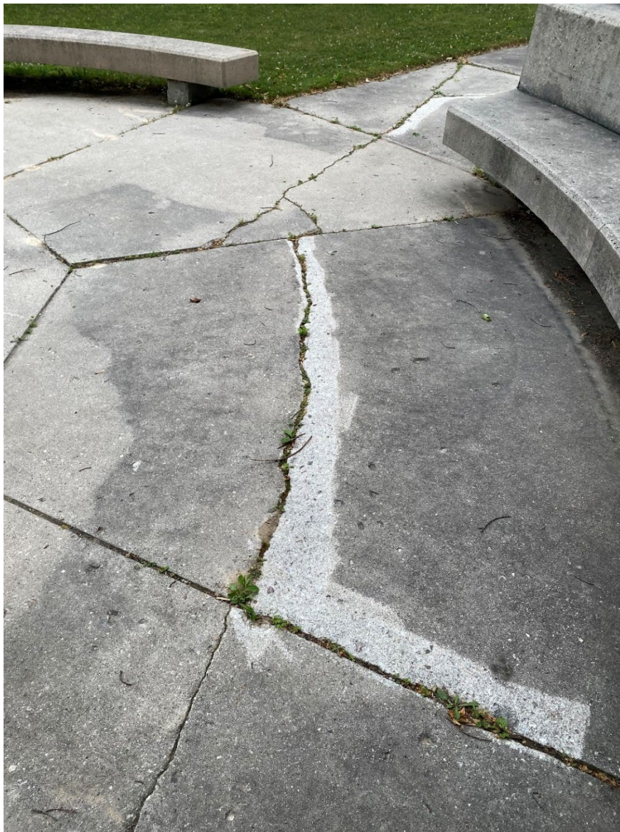
Figure 39: Cracking and settling concrete in courtyard.
