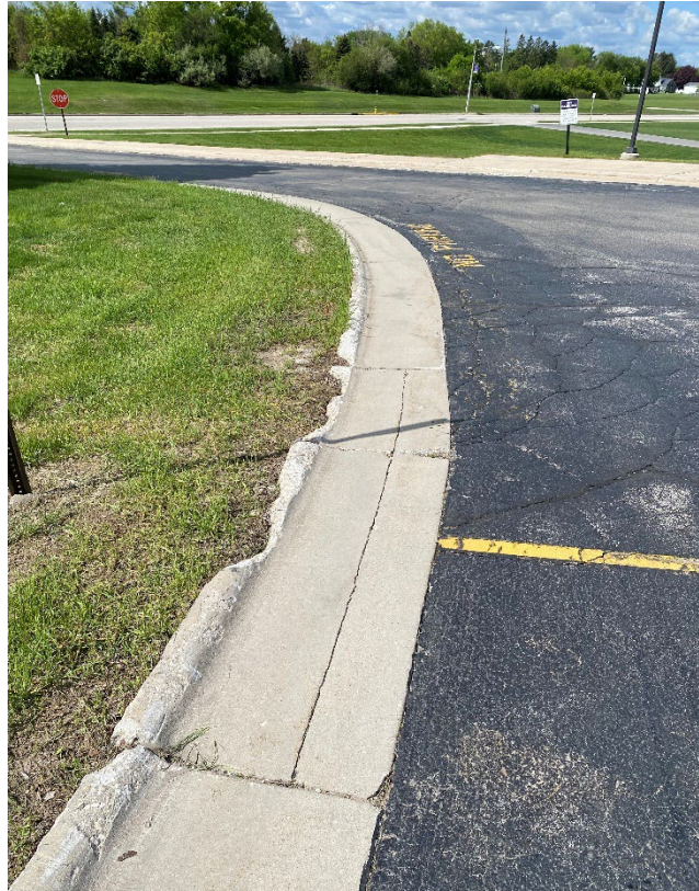
Figure 4: Curb head broken off in Bus/Visitor Parking Loop.
