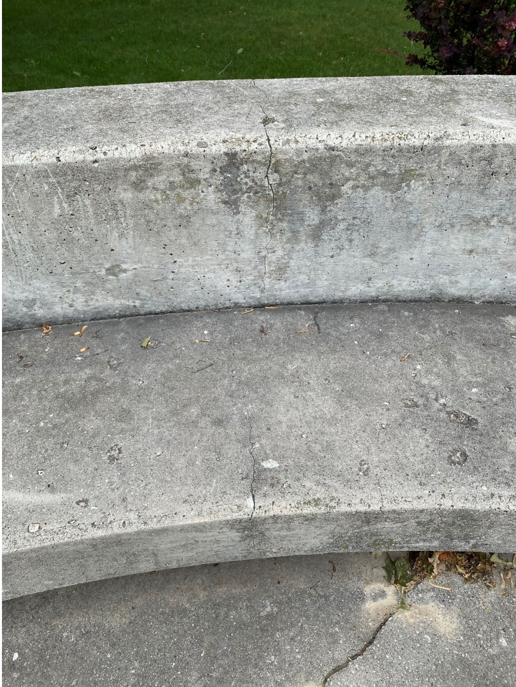
Figure 42: Cracking in circular concrete bench in center of courtyard.
