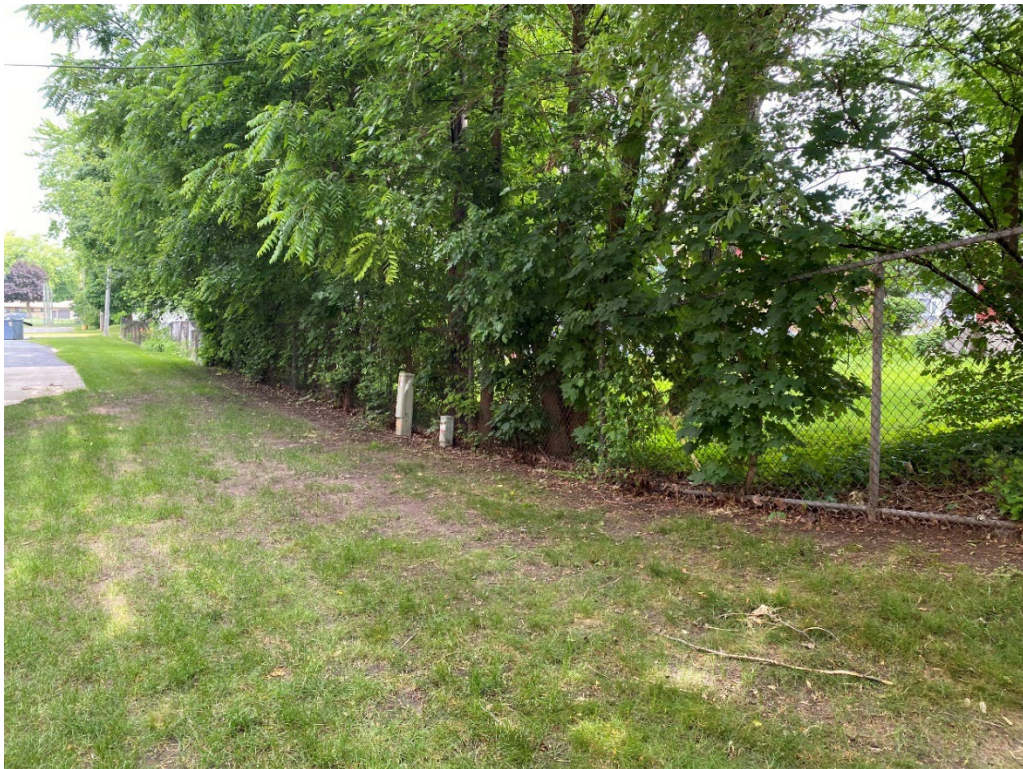
Figure 61: Metal fence on east property line falling over and overgrown with trees.
