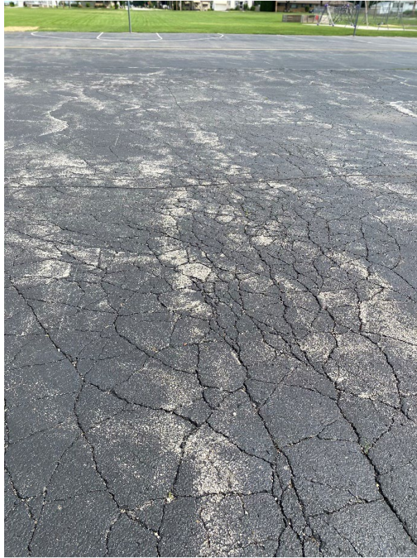
Figure 41: Severe alligator cracking in back play yard.
