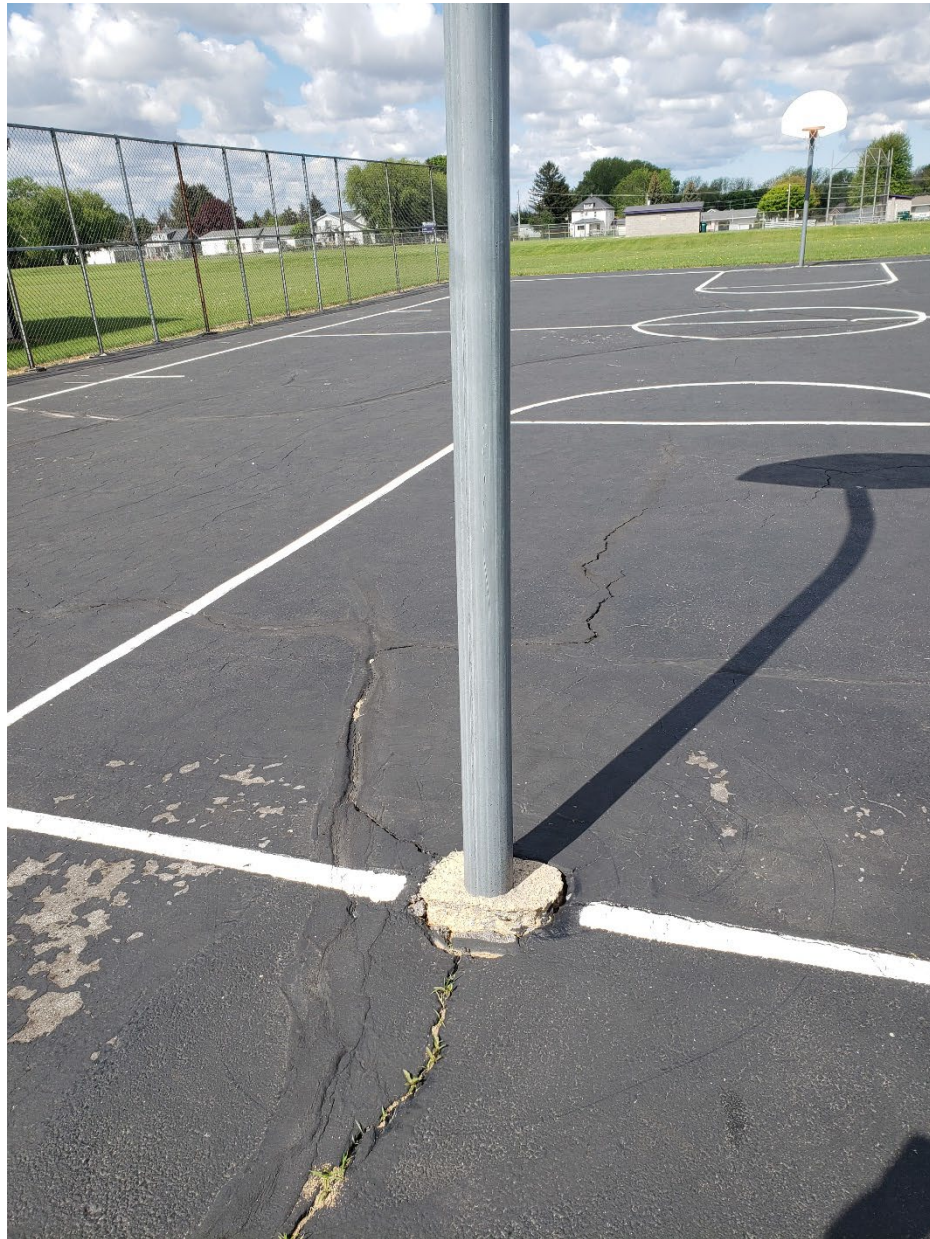
Figure 25: Basketball court with alligator and transverse cracking
