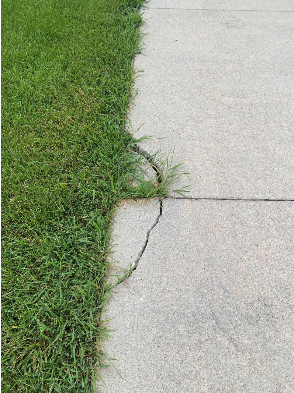
Figure 17: Corners cracked off front center west concrete sidewalk.
