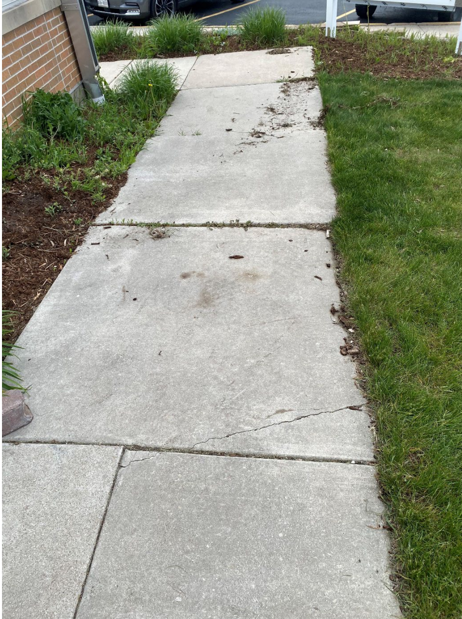
Figure 17: Cracked and uneven sidewalk around greenhouse
