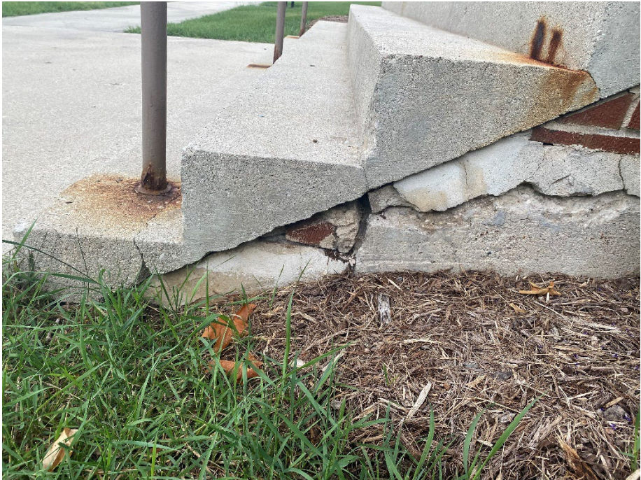
Figure 13: Foundation deterioration of front center west concrete stair.
