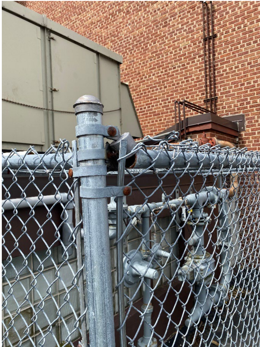
Figure 47: Damaged fencing surrounding mechanical equipment on back side of school.
