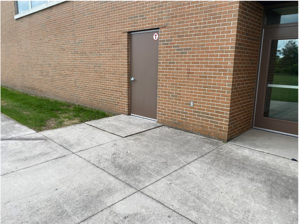
Figure 20: Worn sidewalk and stoop height higher than surrounding pavement on north side of school
