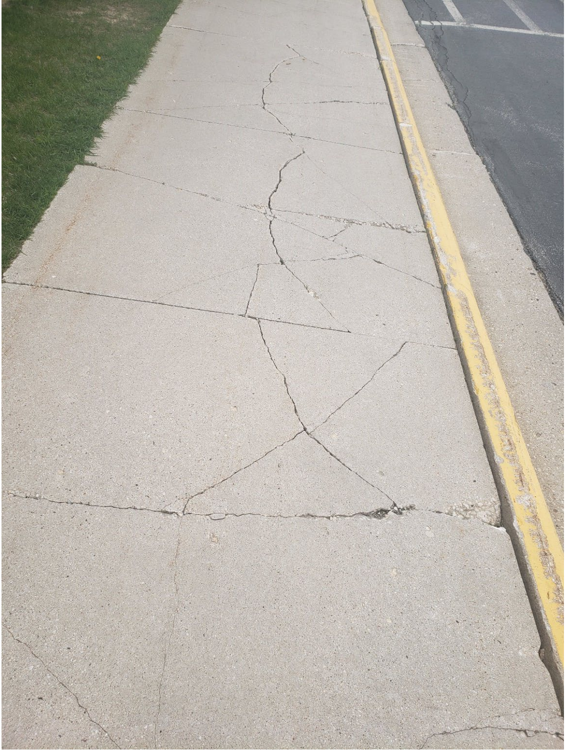
Figure 5: Severe cracking in sidewalk by north doors on west side of school.
