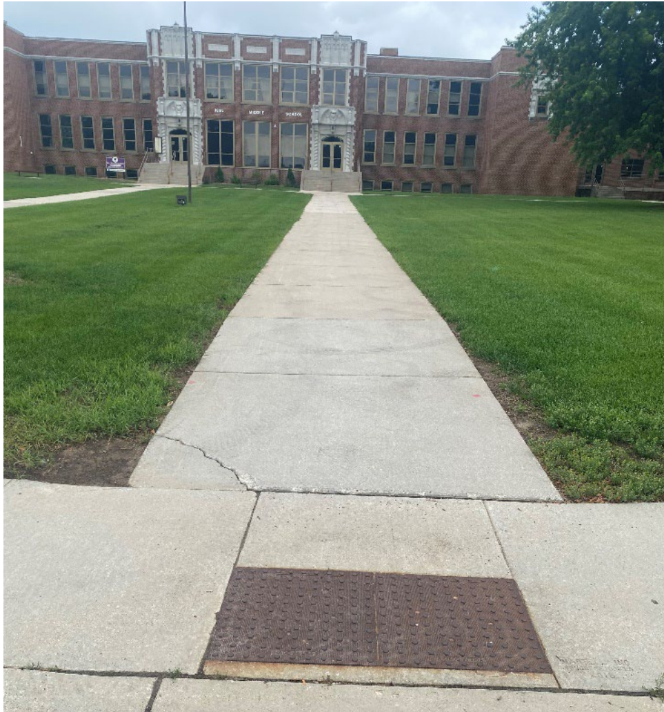
Figure 11: Corner of concrete sidewalk slab cracked off at south slab of center east sidewalk.
