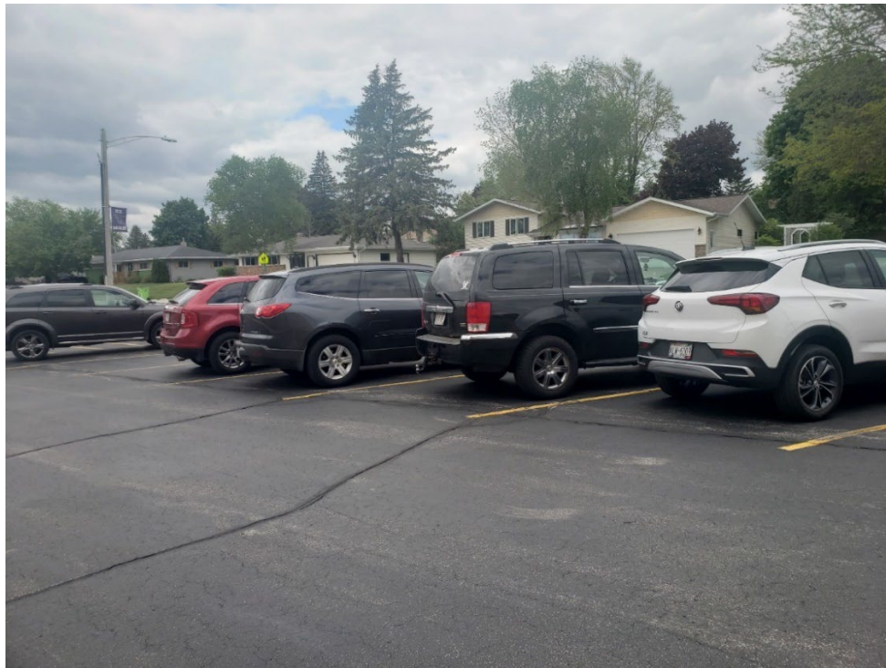
Figure 4: Transverse crack in West parking lot.
