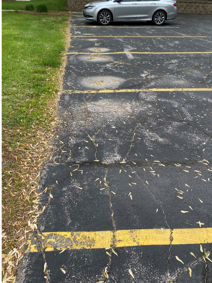
Figure 3: Pavement settling occurring in southeast parking lot.
