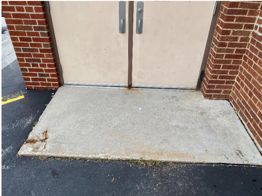
Figure 43: Deteriorating concrete stoop in back play yard.
