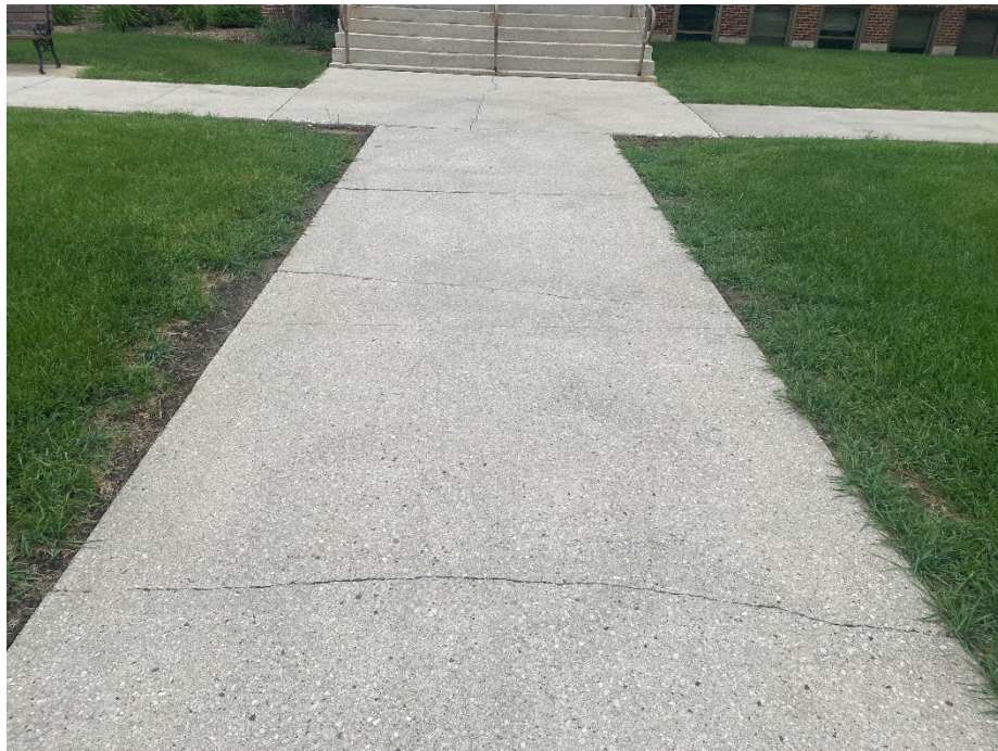
Figure 10: Horizontal cracking in front center east Sidewalk.
