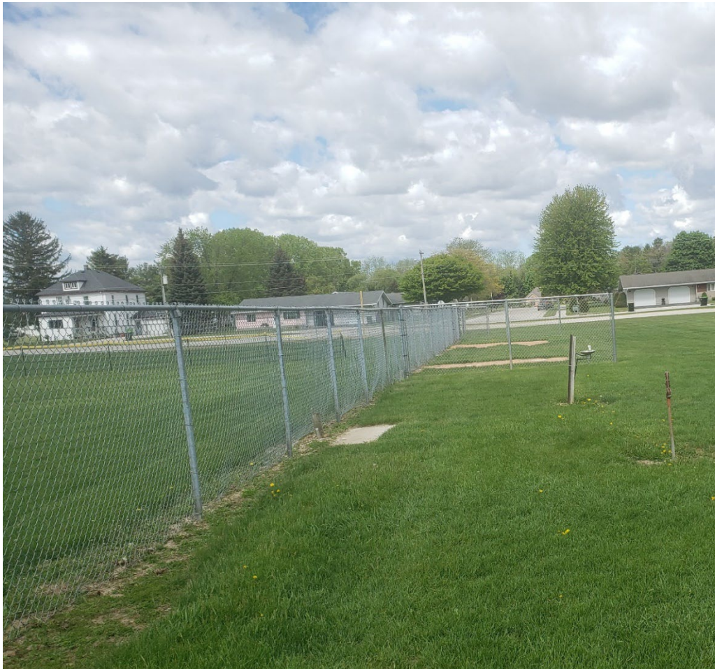
Figure 28: Fencing unraveling at bottom and unattached from posts.
