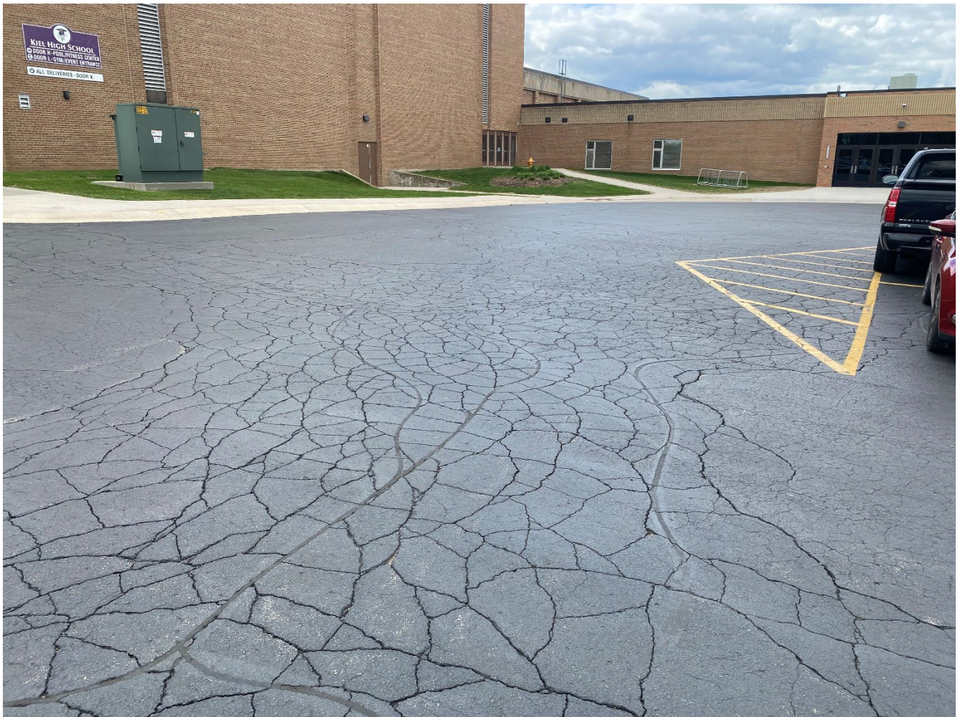
Figure 14: Alligator cracking in Student Parking Lot
