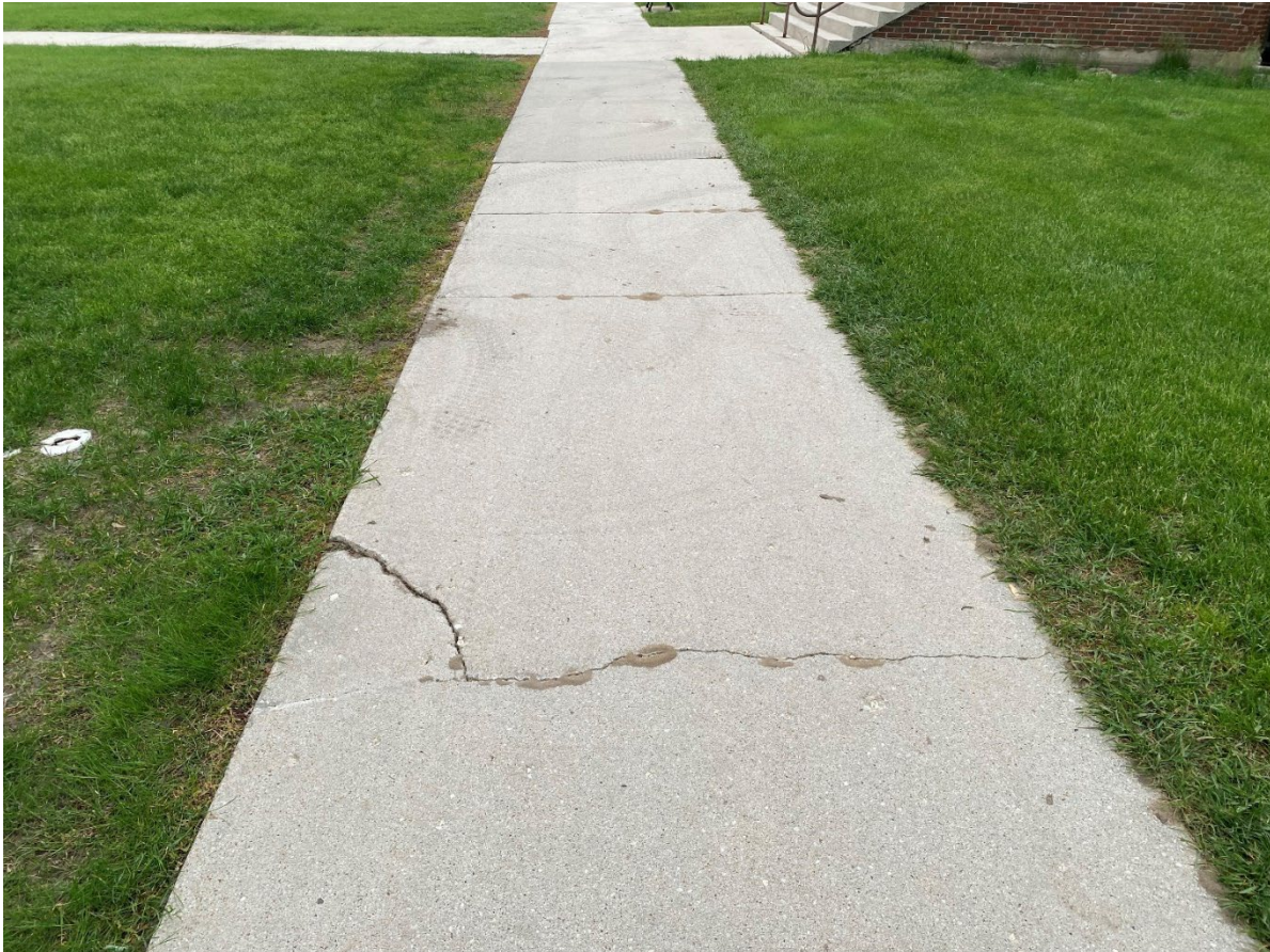
Figure 6: Cracking in east to west sidewalk.
